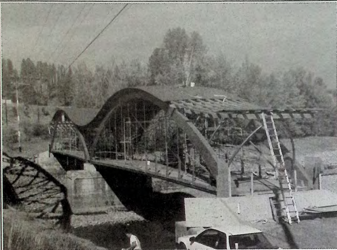
The roofing project on the Bridge of Dreams as it looked on October 8, 2009. *
