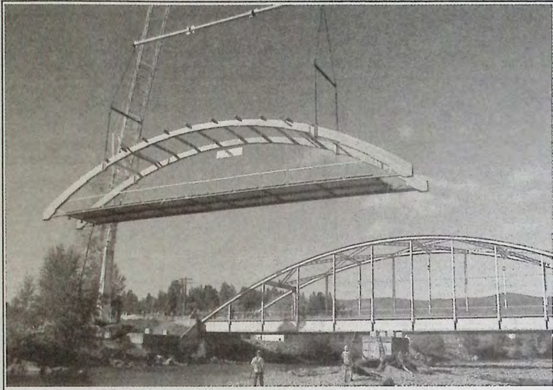
A crane lifts a portion of the Bridge of Dreams in place on September 17, 2009. *
