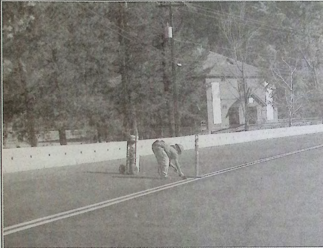
Traffic on Highway 3 near Hedley was down to single lane early this week for shoulder paving, which also required a bit of site preparation prior to the heavy equipment arriving. The delays were not long going either direction. *
