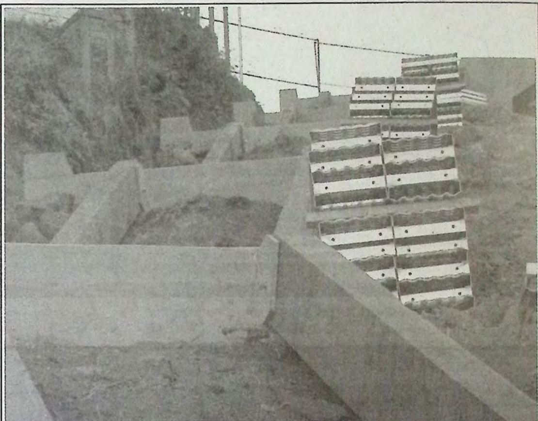
By the time the day was over October 10th, crews had completed the placement of the stringers which linked all the cement landings together on the downtown zigzag project. The stairway is the next step. *
