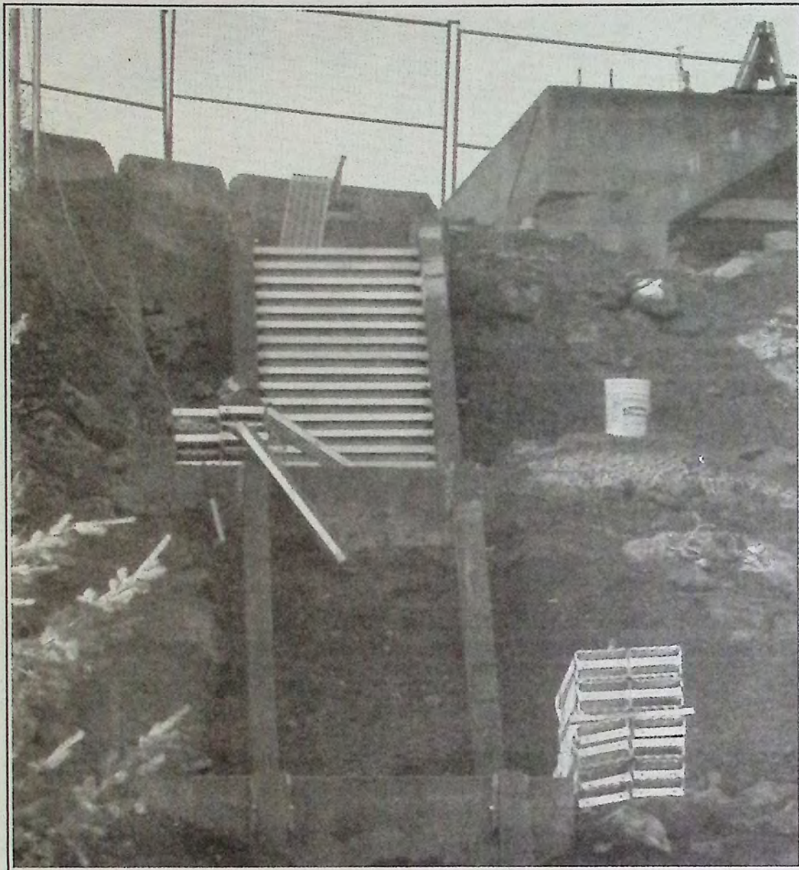
The top set of steps were installed October 15th on the zigzag project with further flights completed during the week. *
