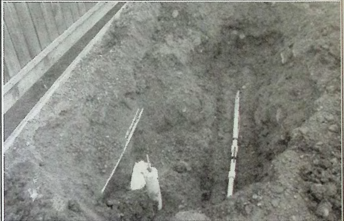
Black tape fastens the underground "Tracer Wire" to the gas line and marks the sleeve put in place to repair the gas line rupture on October 17th. See letter below for details concerning this incident. Photo: Arlene Arlow
