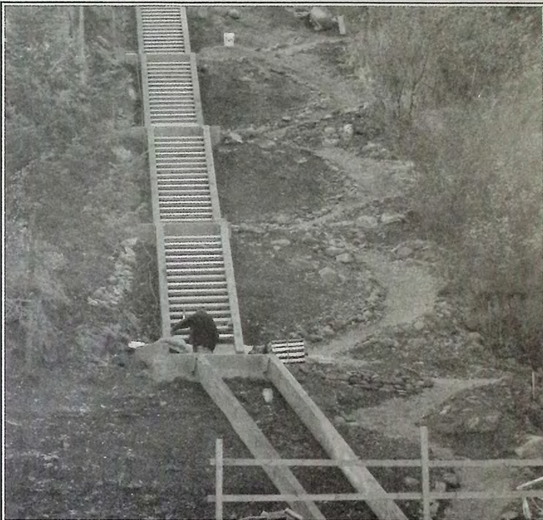
This is how the zigzag project looked mid-week. The dirt path 'zigzag' is very clear to the right of the flights of stairs. *
