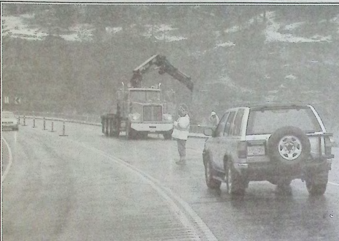
Argo Road personnel use a picker truck the morning of October 23rd to move cement barriers at Yellow Lake that had been pushed out of place by a wayward logging truck. Highway traffic was slowed to one-way traffic in the interests of safety. The cement barricades had done their job: they absorbed the impact of the previous morning's collision and prevented the truck and trailer from careening into the lake. Although the curve was straightened slightly during road construction in 2011, it is still obviously a perilous corner. Drive with caution! Photo: Arlene Arlow
