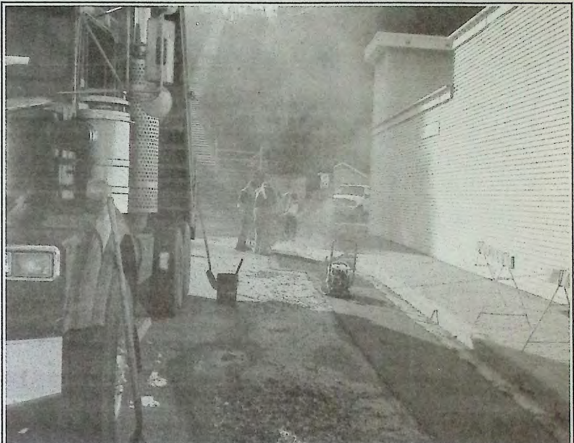
Crews spent October 25th paving the newly created drainage pit and strips along sidewalks on Billiter Avenue near the foot of the zigzag project. There had been no parking there since the project started. Photo: Brenda Engel
