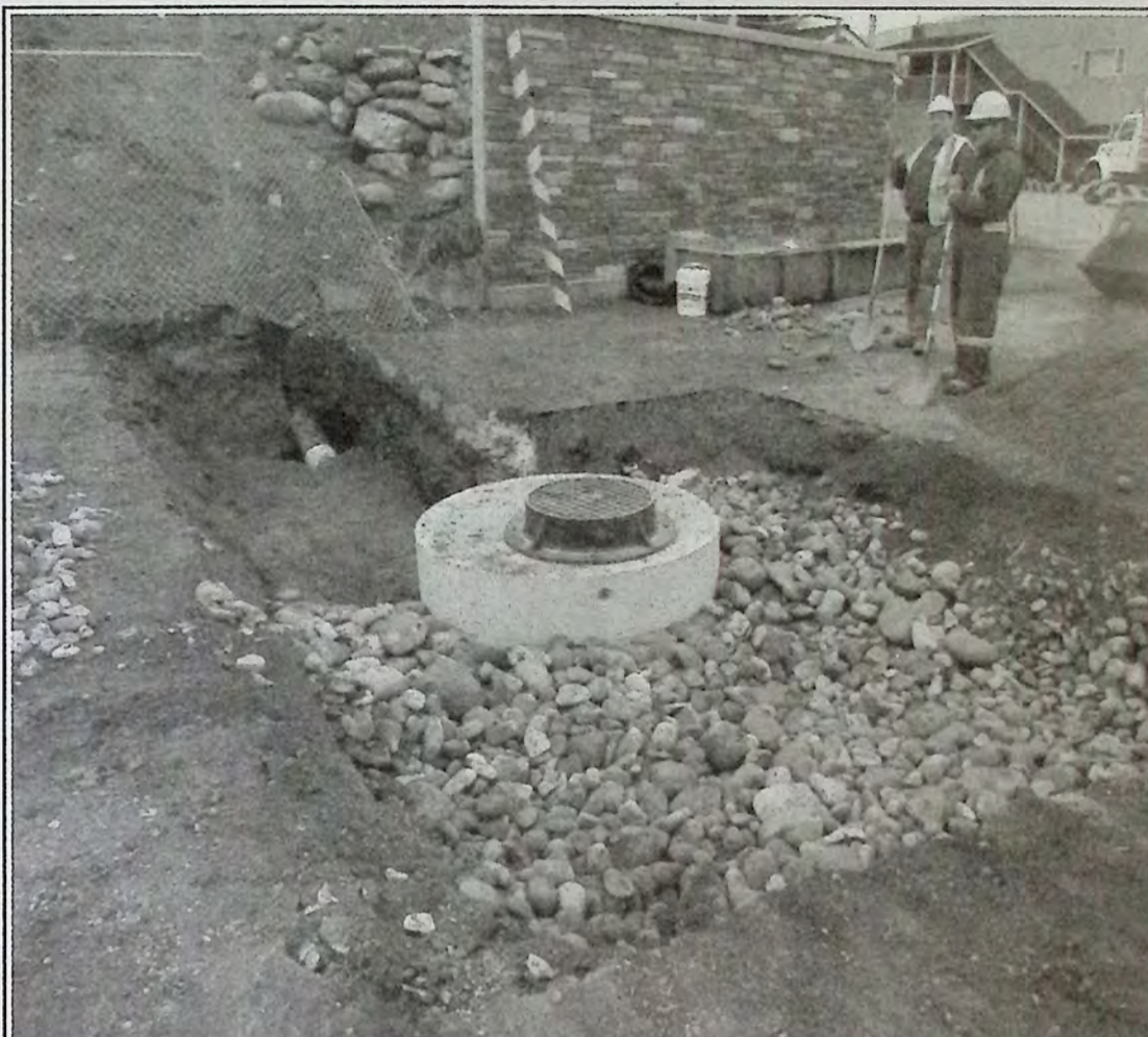
Work on the zigzag project last week focused on correcting the drainage issue. The drain pipe, visible in the back of this pit, was buried the week before running from a catch basin at the top of the project to this location. This work took most of the day October 24th for digging and installing this drainage pit. Photo: Brenda Engel
