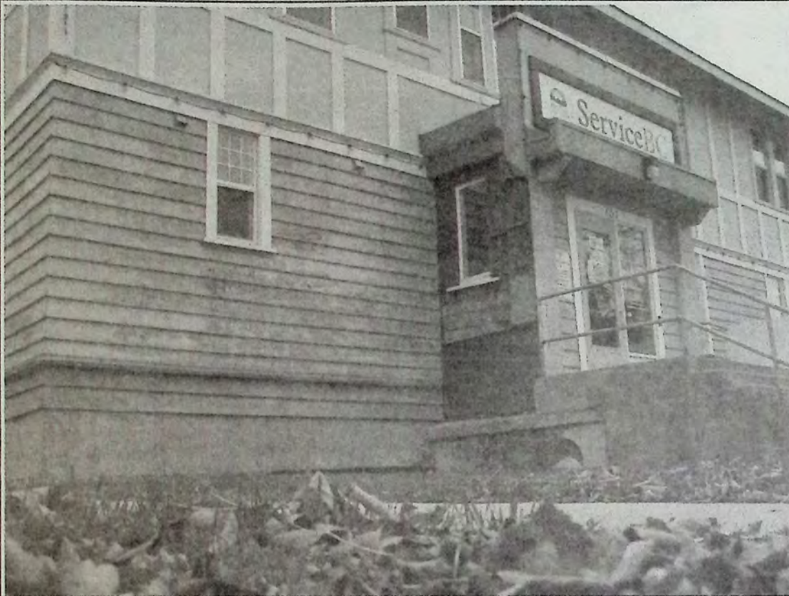
The courthouse building on Vermilion Avenue continues to be the focus of attention as the Town of Princeton proceeds with a structural assessment of the site. It could become the new municipal office. *
