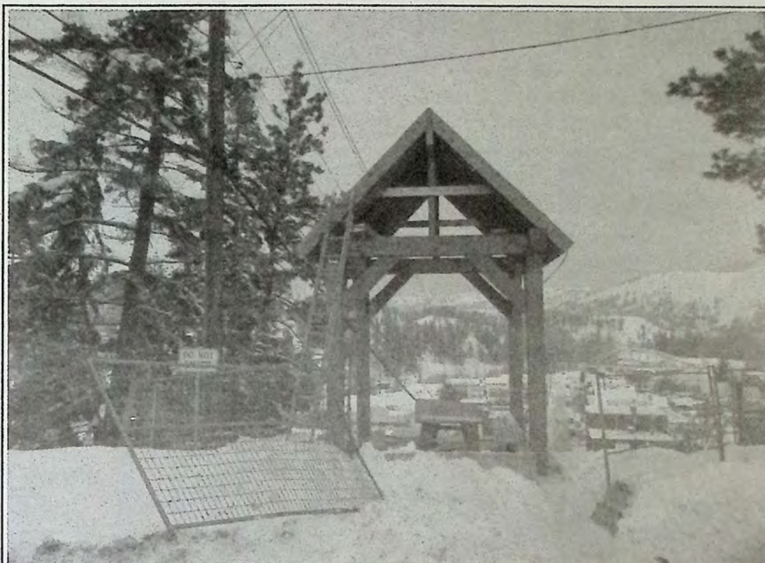
Crews were finishing up the final touches to the roof of this gazebo-style entrance located at the top of the zigzag last week. Although it is clearly marked below with a 'No Trespassing' sign, residents have been using it 'as is.' Handrails will not be installed until spring which will pretty much bring the project to an end. Photo: Brenda Engel
