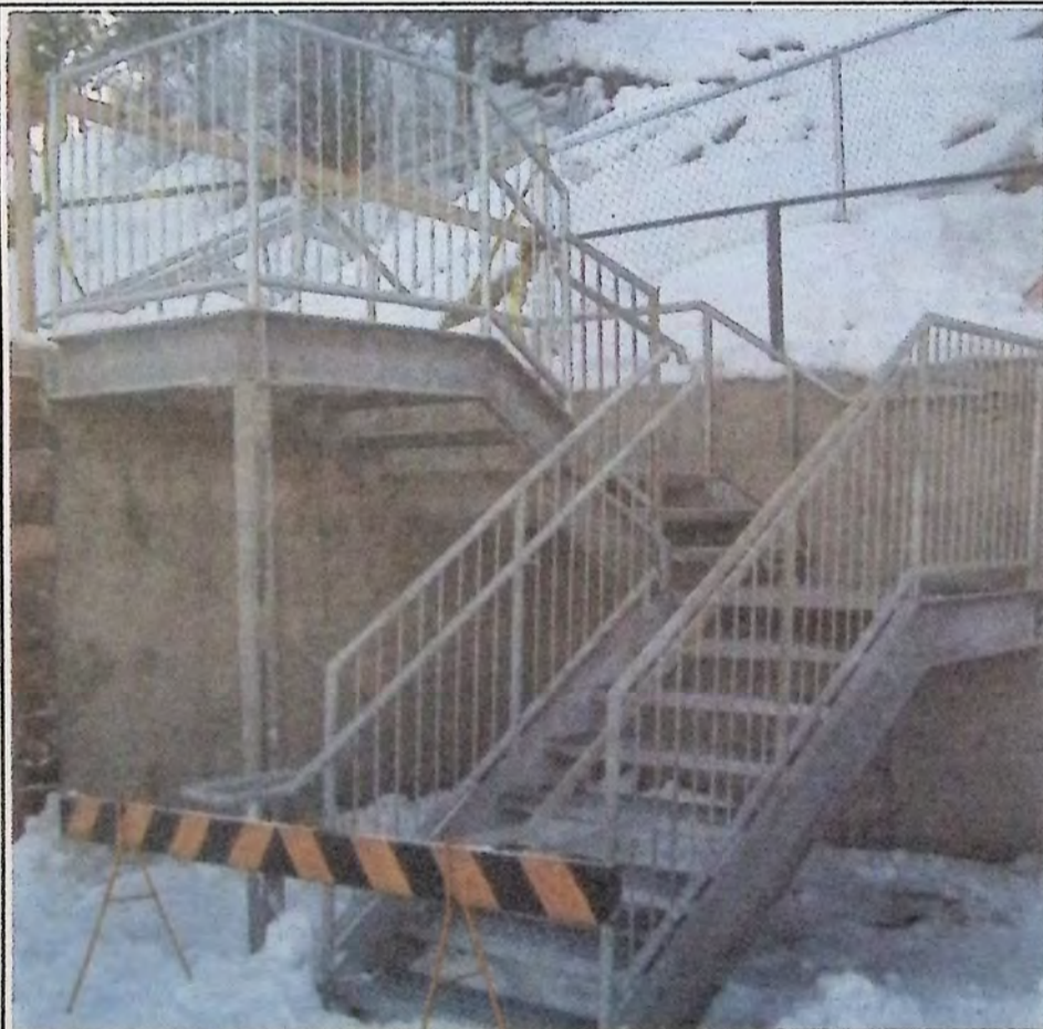
The downtown zigzag project now has a proper stairway entrance at the foot of Billiter Avenue. This was installed early February 2nd, but is not 'officially' open yet for regular use. *
