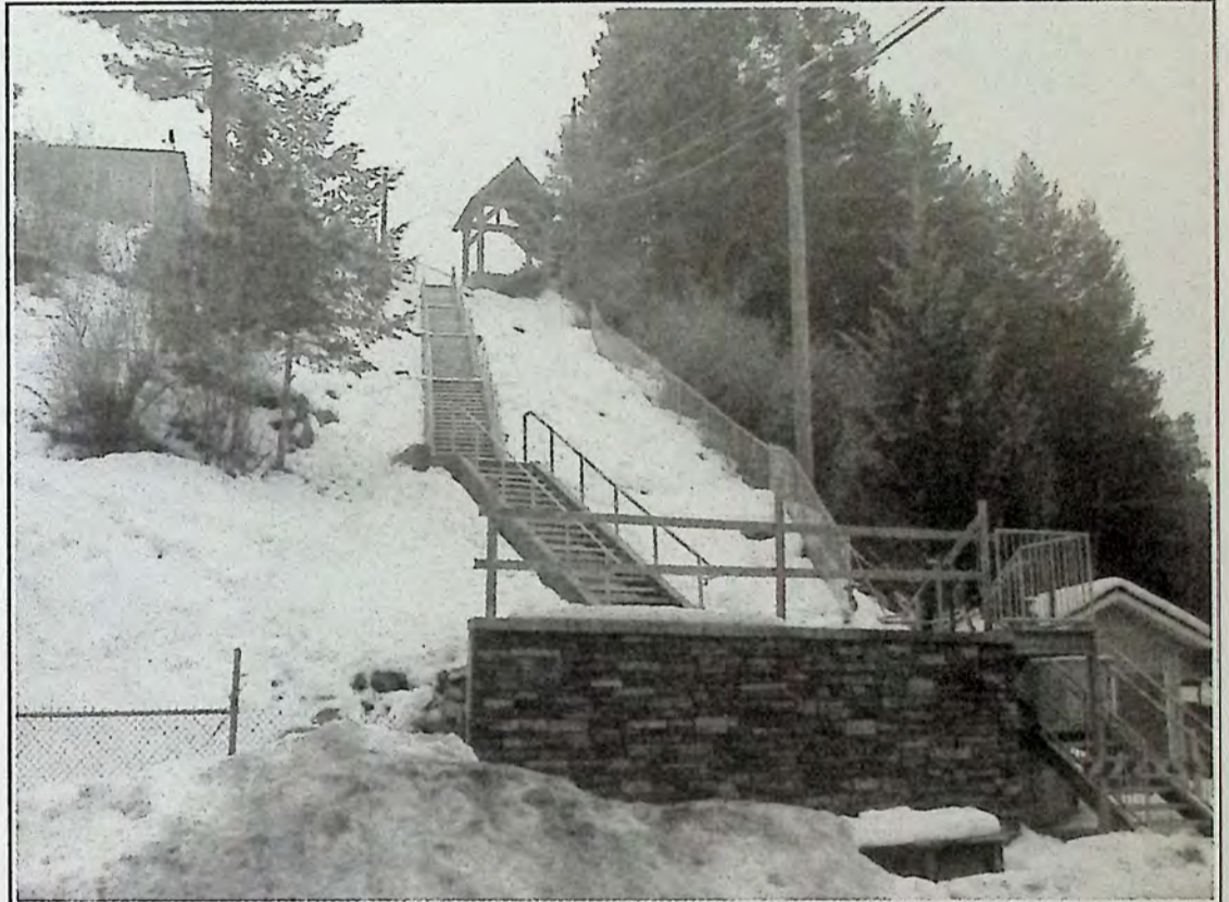
Handrails were installed on the zigzag February 14th, but it is still not open to the public. *
