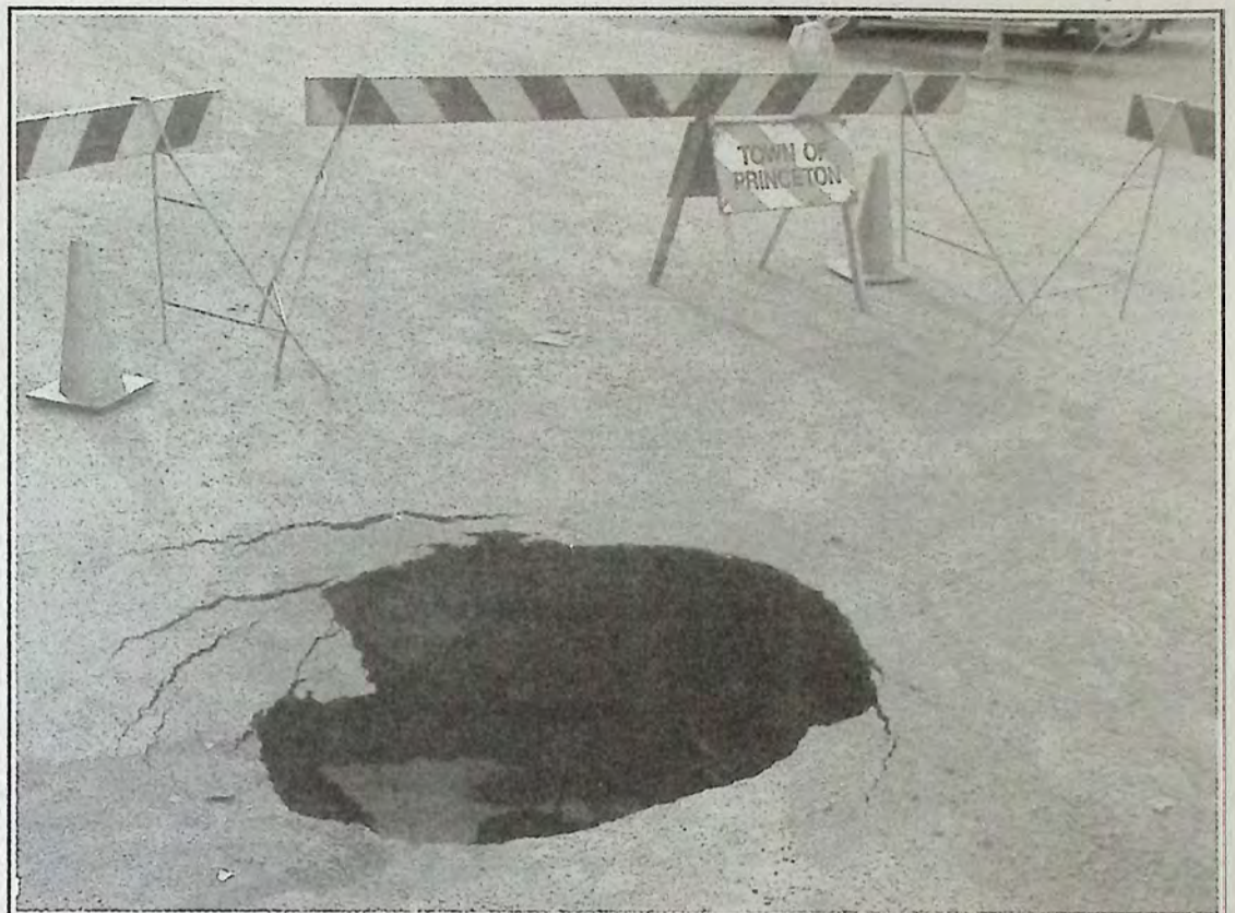
A sinkhole has developed in the alley that runs behind Shoppers Drug Mart on Bridge Street. Photo: Brenda Engel
