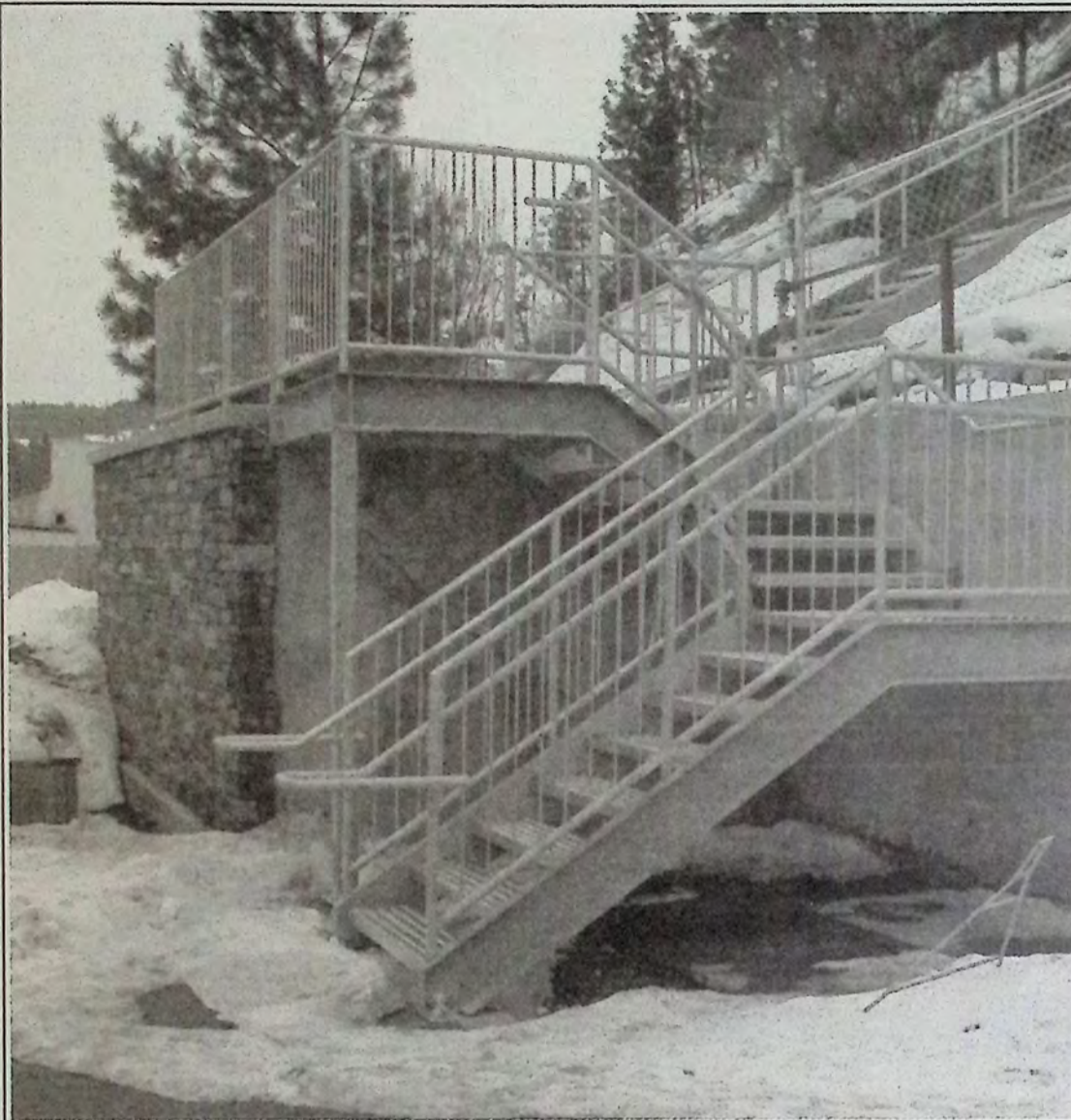
Although it was only supposed to take a matter of weeks, the downtown zigzag project has taken months to complete due to a series of glitches that popped up along the way. Guardrails at the top of the retaining wall were installed March 5th bringing the project one step closer to being completely finished and open to the public. *
