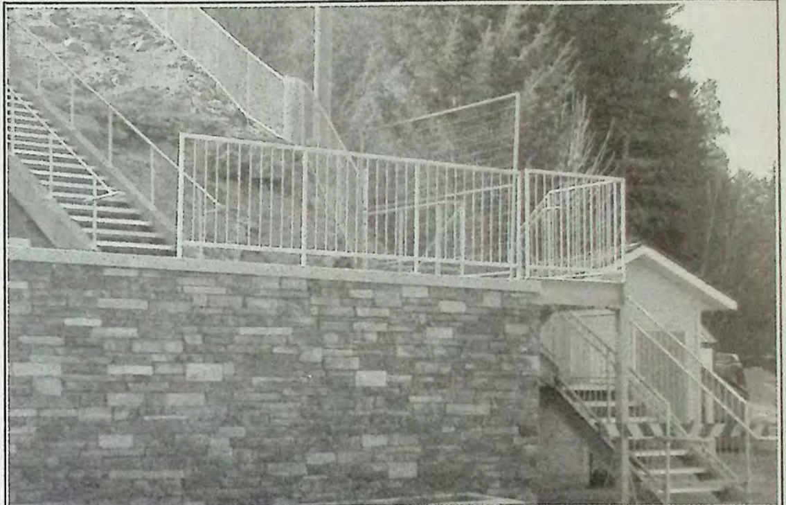
A large wire gate has been attached at the top and bottom of the zigzag to block access until the project is completed. Some residents were hopping over the two-by-four barriers to use the route. Photo: Brenda Engel
