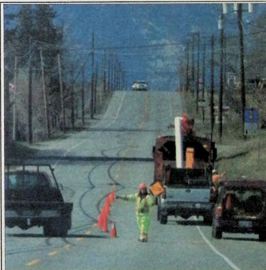
Fortis crews were busy trimming trees away from power lines along Highway 3 March 25th. Traffic experienced the normal delays related to single-lane traffic just east of Keremeos. Photo: Arlene Arlow
