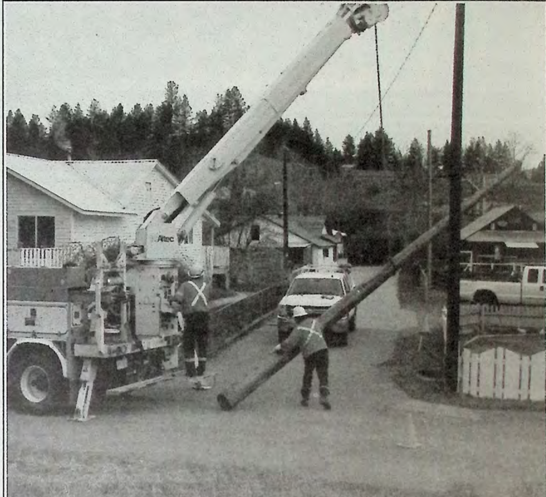
FortisBC's Jason Earle and Aaron Gould show their professional skills with a power pole replacement that saw a them place a new pole along Waterfront Avenue on April 4th with speed and efficiency. Photo: Brenda Engel
