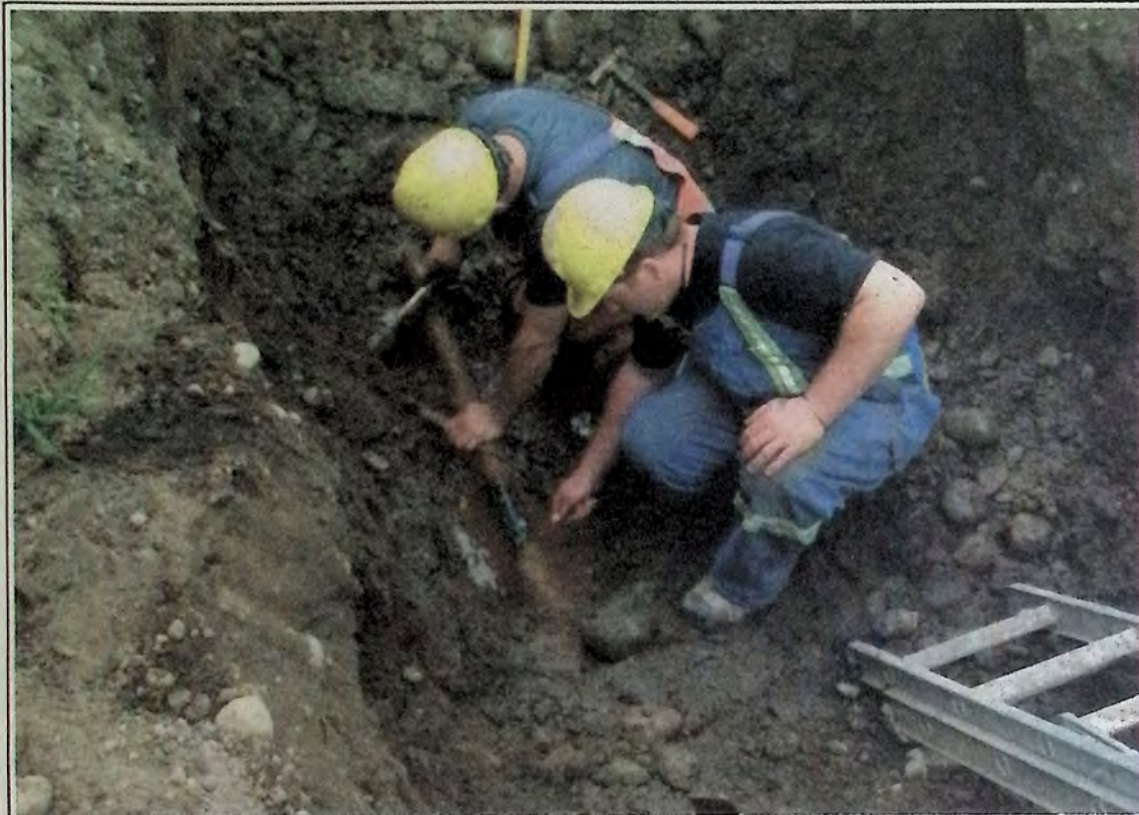
Princeton town crew repair a water leak April 25th in the lane behind Cedars Motel. It is the fourth leak repair fixed in as many days. Interim Public Works Manager Bruce Hamilton says old pipes are to blame. Photo: Brenda Engel
