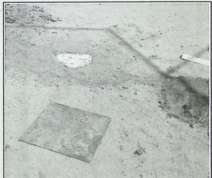
Some of the work done last week at Memorial Park was repairs to one of the ball diamond in fields. This photo shows realignment work on home plate which saw it relocated (it was to the right). Photo: Brenda Engel
