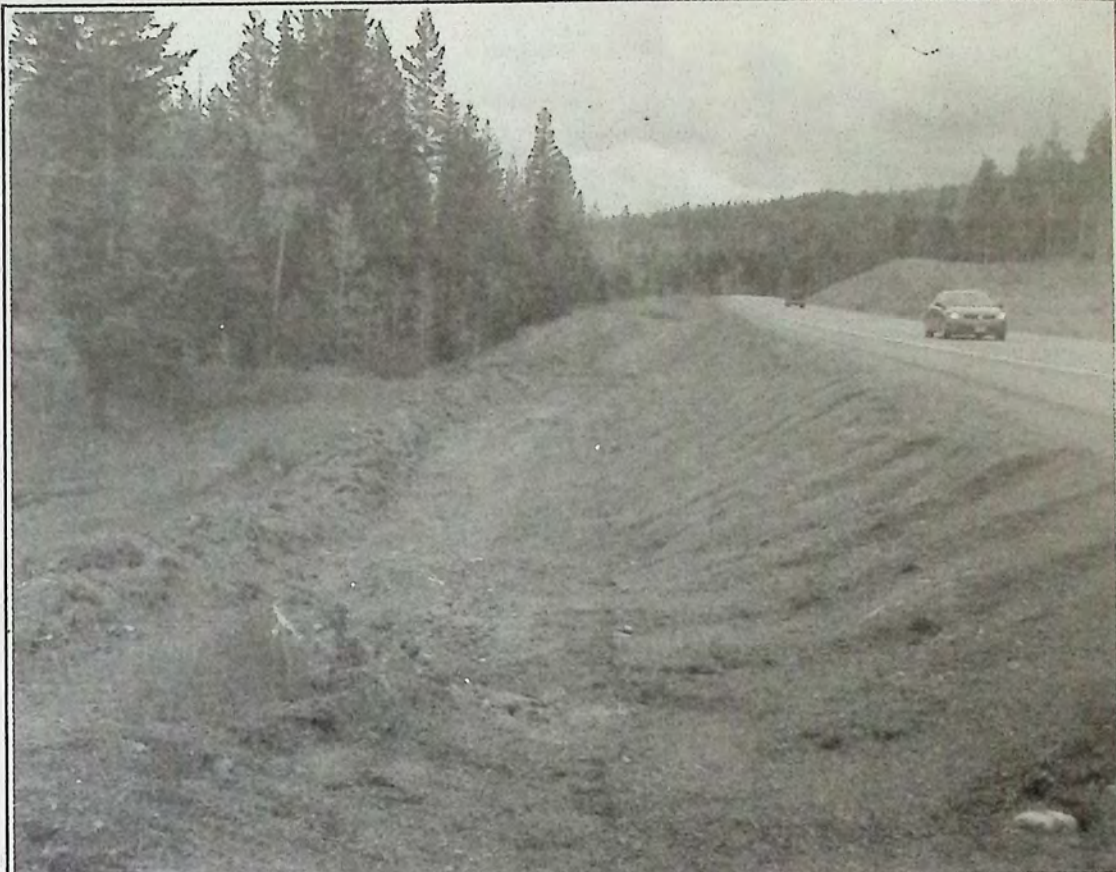
The four-lane project West of Princeton continues to show signs of progress.*
