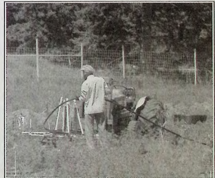
It takes two good men to lay irrigation line (and a tractor and a four-wheeler). Sunday June 9th was all about farming in and around Keremeos. The other worker in this duo (who is also a co-owner of the property) was pulling the irrigation line along with his four-wheeler. Once the line is placed, it needs to be hooked up to the system and buried. The property being put into production is just north of Keremeos on Highway 3. The previous owner had the land planted to hay. Hay introduces all kinds of nutrients into soil so the first crop from this newly-planted orchard will require little fertilizer and will likely be a bumper crop. The new owners and their employees are working hard to change the hay land into orchard. Photo: Arlene Arlow
