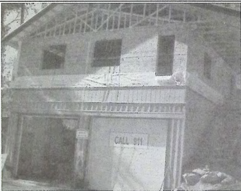
When in doubt, call 9-1-1! Hayes Creek Fire Hall construction site. Photo: Rob Miller
