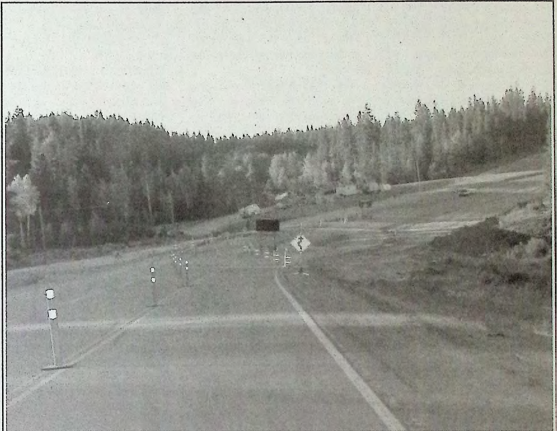
They weren't kidding when they said the traffic pattern changes! Construction continues on the 4-laning project on Highway 3 West of Princeton. Expect minor delays daily until 6:00 PM.*
