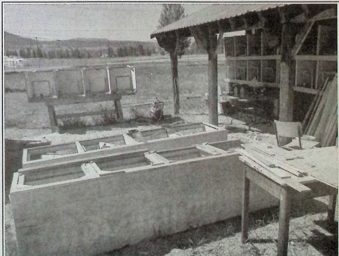
Here's a look at the project of replacing the poultry display area with new coops partway through the construction phase. The improvements have greatly enhanced the area. - photo submitted
