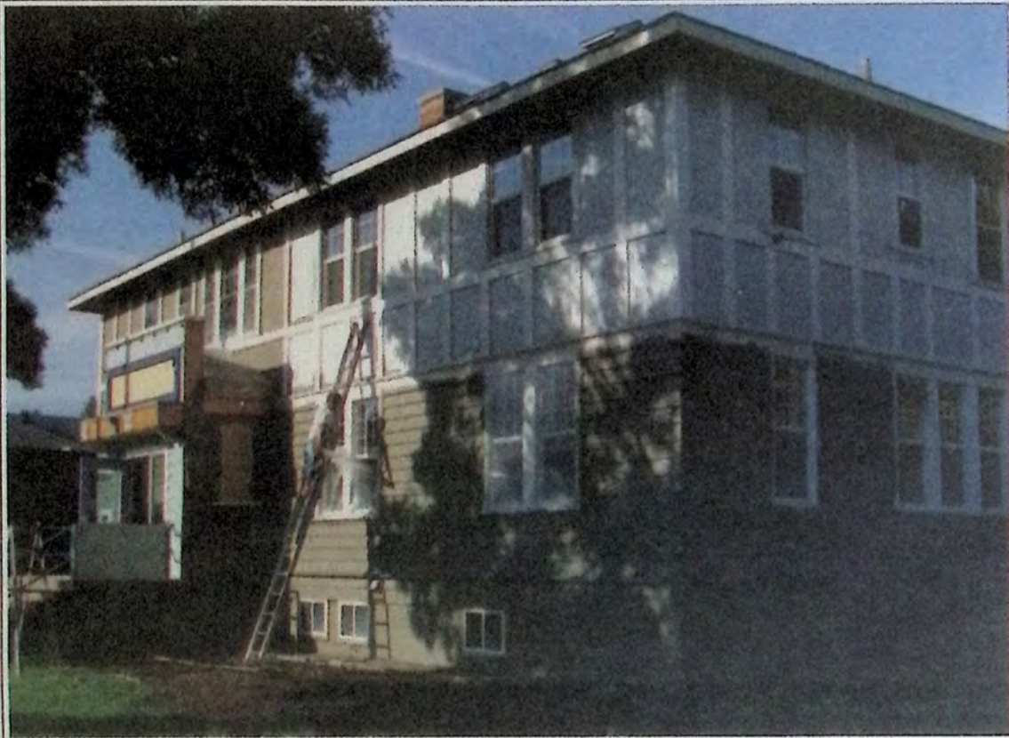
The Courthouse building on Vermilion Avenue continues to get renovated so that it can become the new Town Hall. The exterior received a serious face lift with a new paint job last week. Here's how it looked early on September 20th. *
