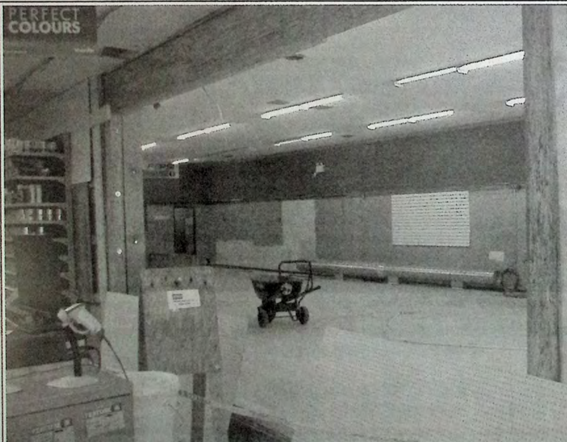
The view from the present Home Hardware looking into the new expansion area. With talk around town related to concern over empty storefronts, this is one positive business forging ahead and investing into the community. *
