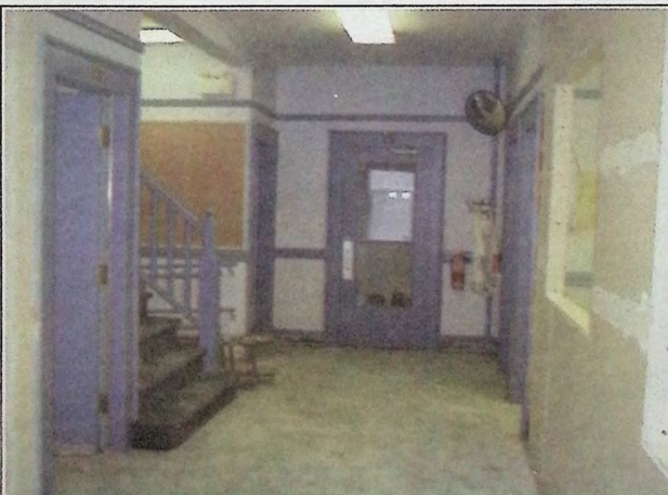
Not a lot of interior structural changes have taken place. To the right of the frame will be the majority of administrative services. The stairs to the left will continue to access court services. *
