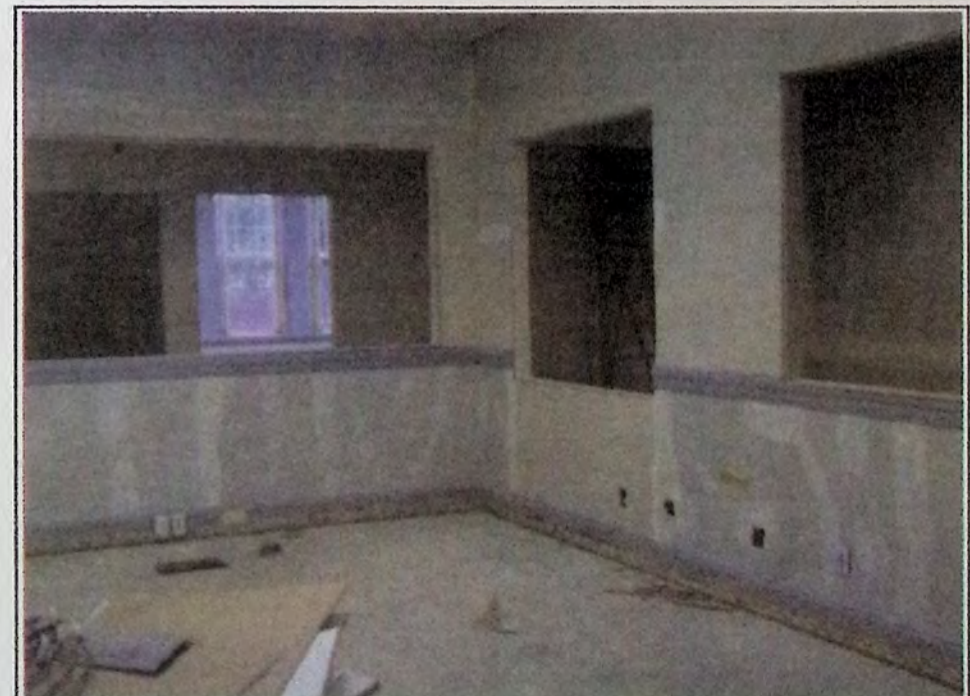
The view from inside the main office. The hallway leading to the left is to handicap access at the rear of the building. Note the lowered window in the centre for wheelchair users. *
