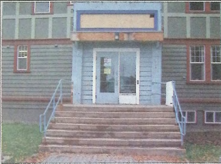
Work should have started on changing the main entrance to the new Town Hall by the time you read this. The new entrance will see covered steps, new railings and more improvements. *
