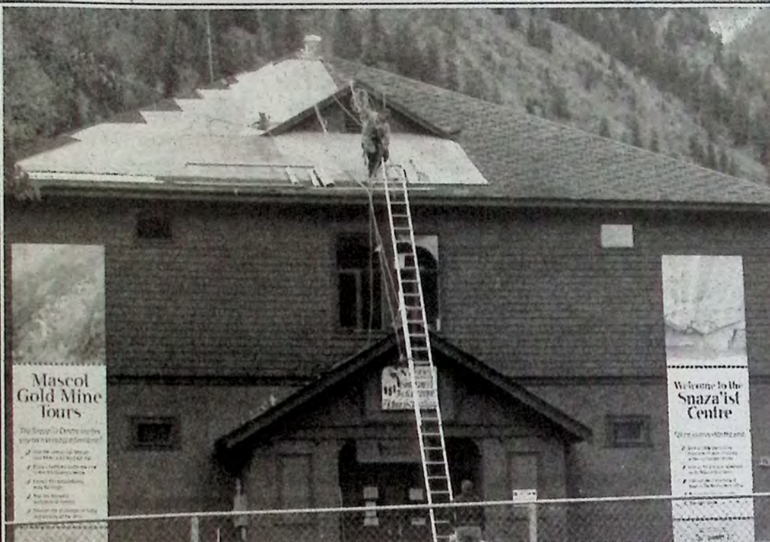
The Snaza'ist Centre in Hedley is getting a much-needed new roof. The ropes over the peak of the roof are testament to the safety measures that roofers need to take so that they don't fall off. Photo: Arlene Arlow
