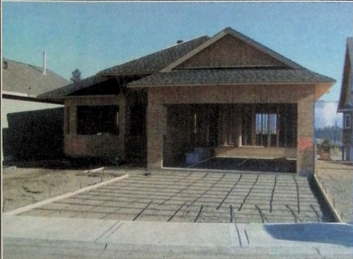
With all the talk around town centering on high rents and empty storefronts there are a lot of positive signs in and around Princeton. This is one of two new homes currently under construction on Copperhead Road. *
