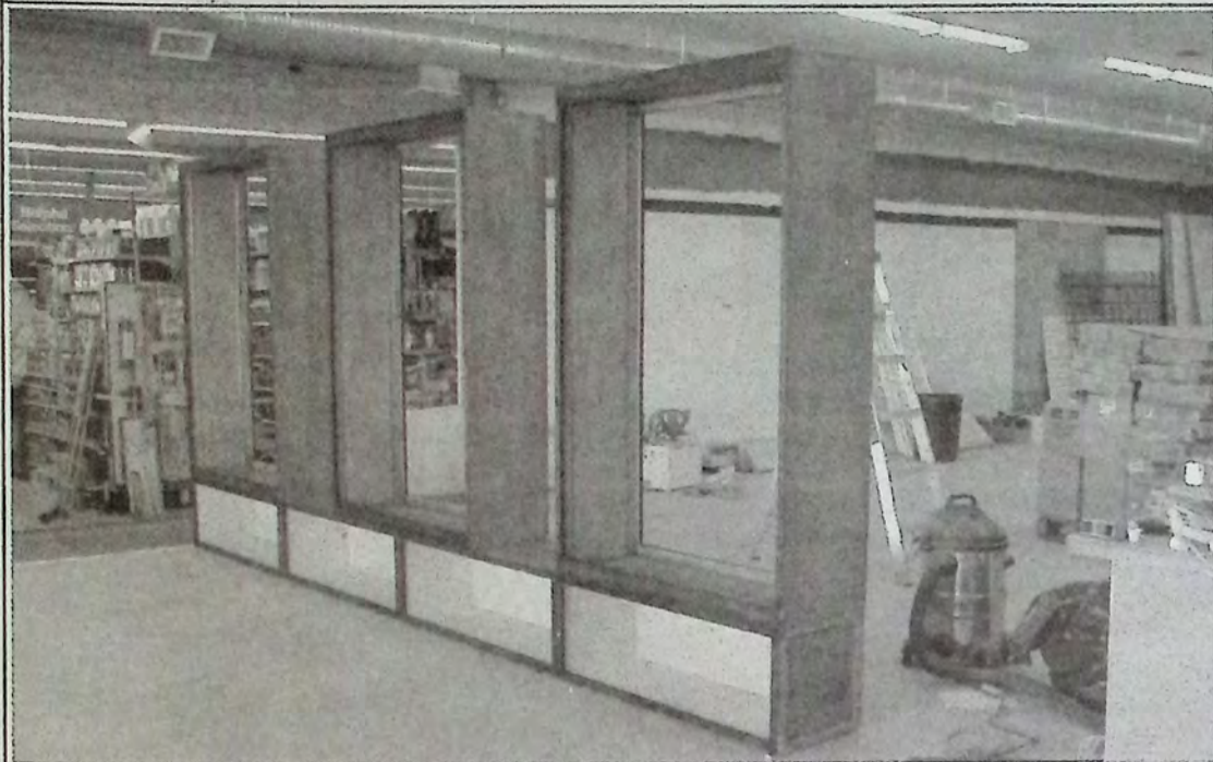
These giant shelves took Princeton Home Hardware Owner/Manager Peter Rubingh two days to build and will become the front window display in the expanded area of the hardware store. Watch for changes daily this week. *
