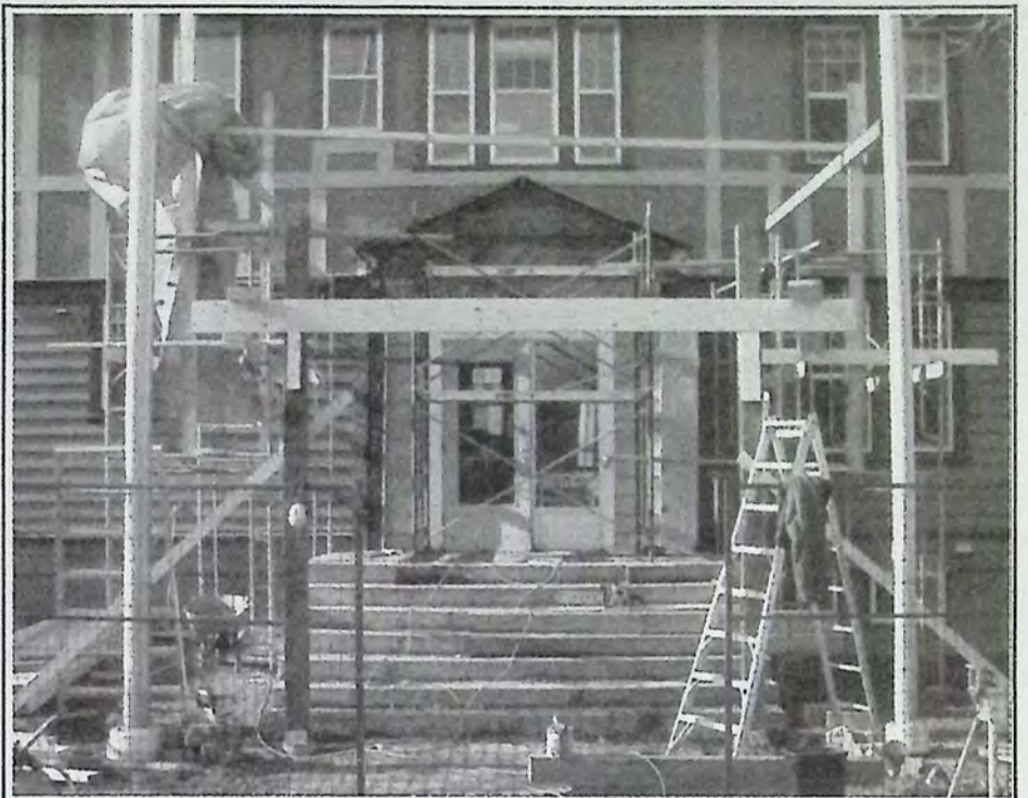
Framing of the new entrance to the 'new' Town Hall took shape November 8th. *
