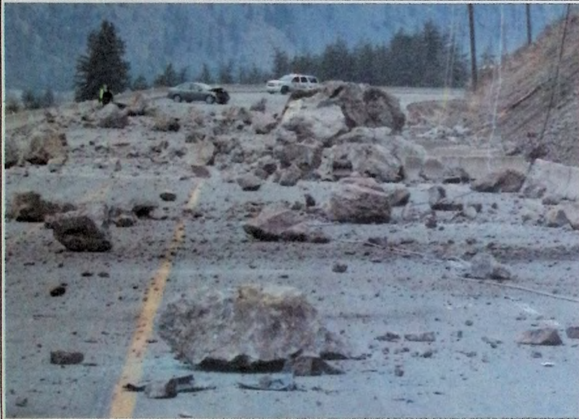
Rocks and debris came crashing down on Highway 3 shortly after 12 Noon Monday, January 27th at a location a short distance west of Keremeos closing the route to all traffic for most of the week. Photo: Brenda Engel
