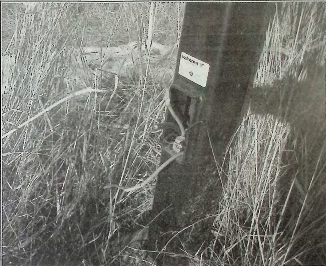
After closer inspection we discovered why some of the lights along the Trans-Canada Trail don't go on at night. It appears that someone doesn't like the way they brighten up the area near Burton Avenue for some reason. *
