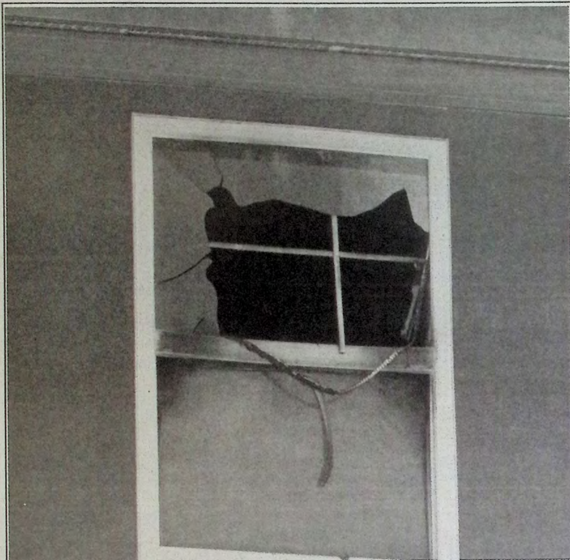
It would appear that the glass in this window is blown outward. The top of the window has a purple residue. The powder-like substance on the inside of the glass may be from the use of a fire extinguisher. The fire on the evening of February 1st started in an upstairs suite of the Riverbed Bistro in Keremeos. The fire investigator and an RCMP officer were inspecting the scene during daylight hours the day after the fire. The structural integrity of the building is intact because firefighters contained the blaze quickly. Photo: Arlene Arlow
