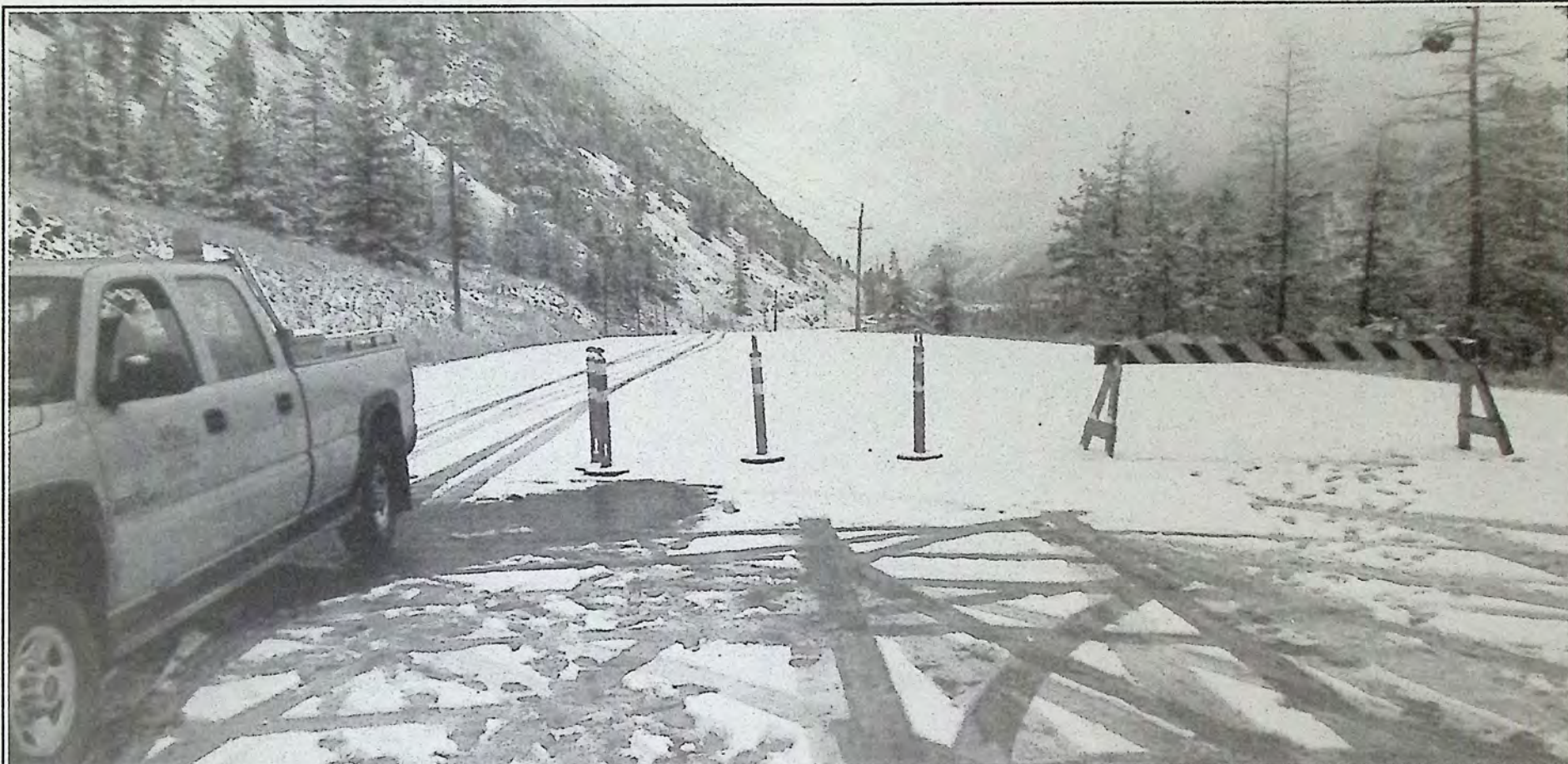
This was the view residents saw at the Princeton end of the section of Highway 3 that was closed to all traffic following a rock slide January 27th. Only two of the four lanes are open at this time. *
