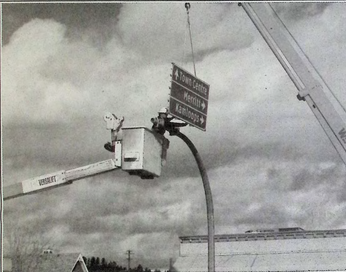
Highways crews spent part of February 12th installing new directional signs at major intersections and along Highway 3 in Princeton. The new, updated signs were a welcome sight for many as they were in need of replacement. *
