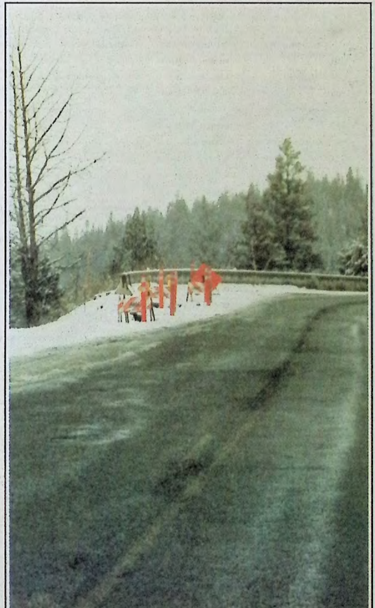
A washout part way up 'Burns Hill' north of Allison Lake on Highway 5A cut the two-lane stretch down to a lane and a half. Photo: Bob Marsh
