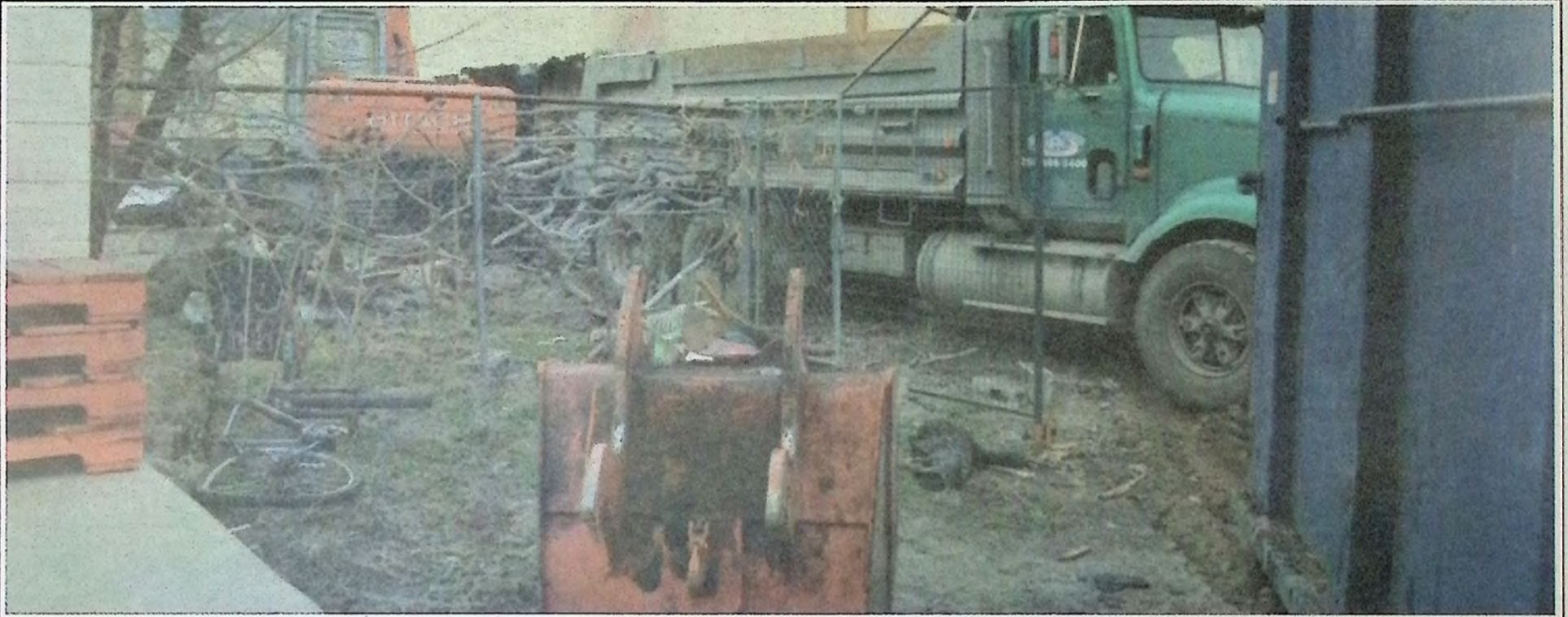
Soon it will be but a memory: cleanup has commenced at the site of the structural fire February 3rd in Keremeos. The older building along the main drag was completely gutted just after midnight February 3rd. The fire is not considered suspicious, having started accidentally in the living quarters at the back of the building. Another structural fire the same weekend in Keremeos occurred at the Riverbed Bistro. That fire was deemed suspicious and is still under investigation. Photo: Arlene Arlow
