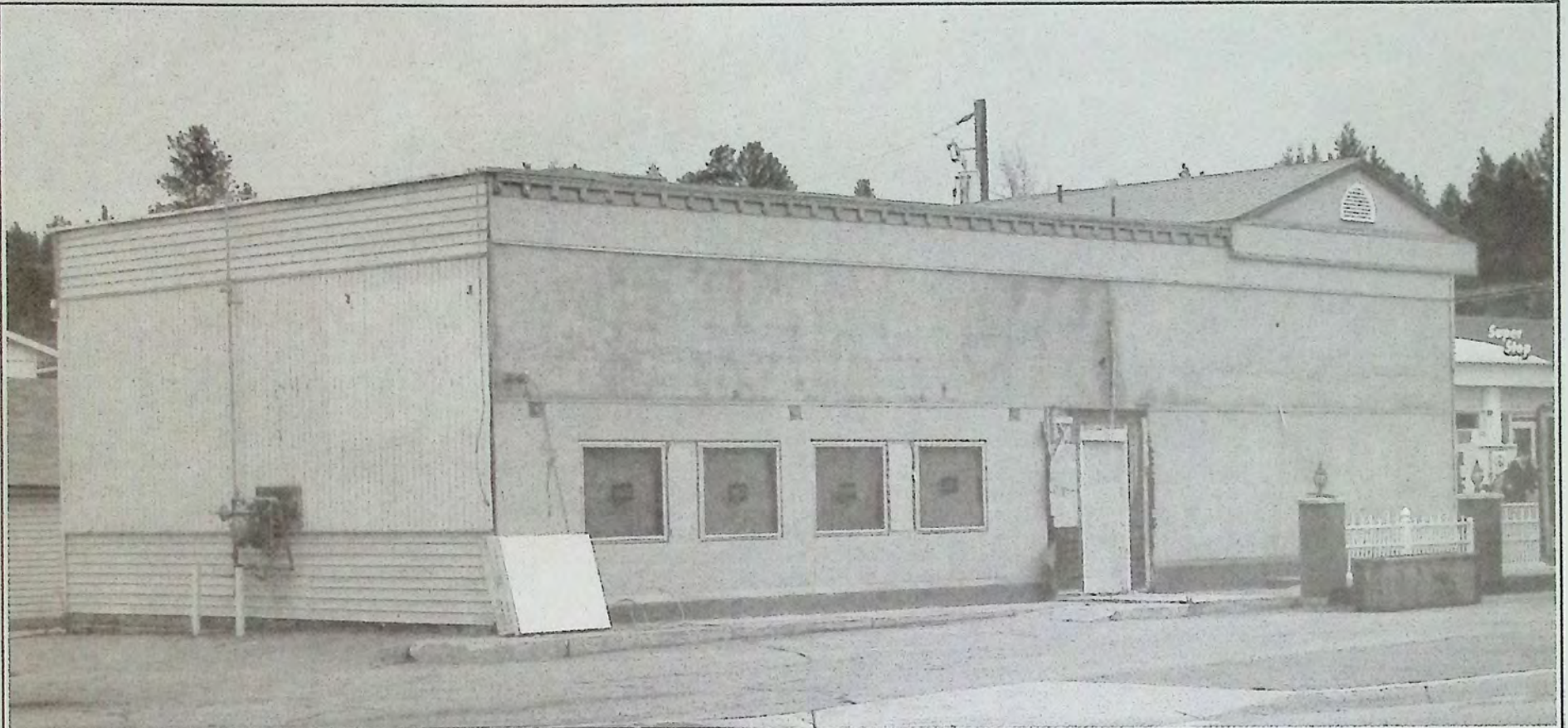
When they said they were giving it a face lift they weren't kidding! The former Santo's Pizza building has been getting renovated and last week it looked like this! Photo: Brenda Engel
