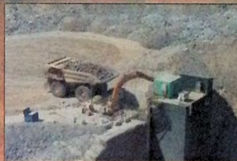
Ore which enters the primary crusher will be further reduced in size by the secondary crusher before it is sent into the SAG mill for grinding.
