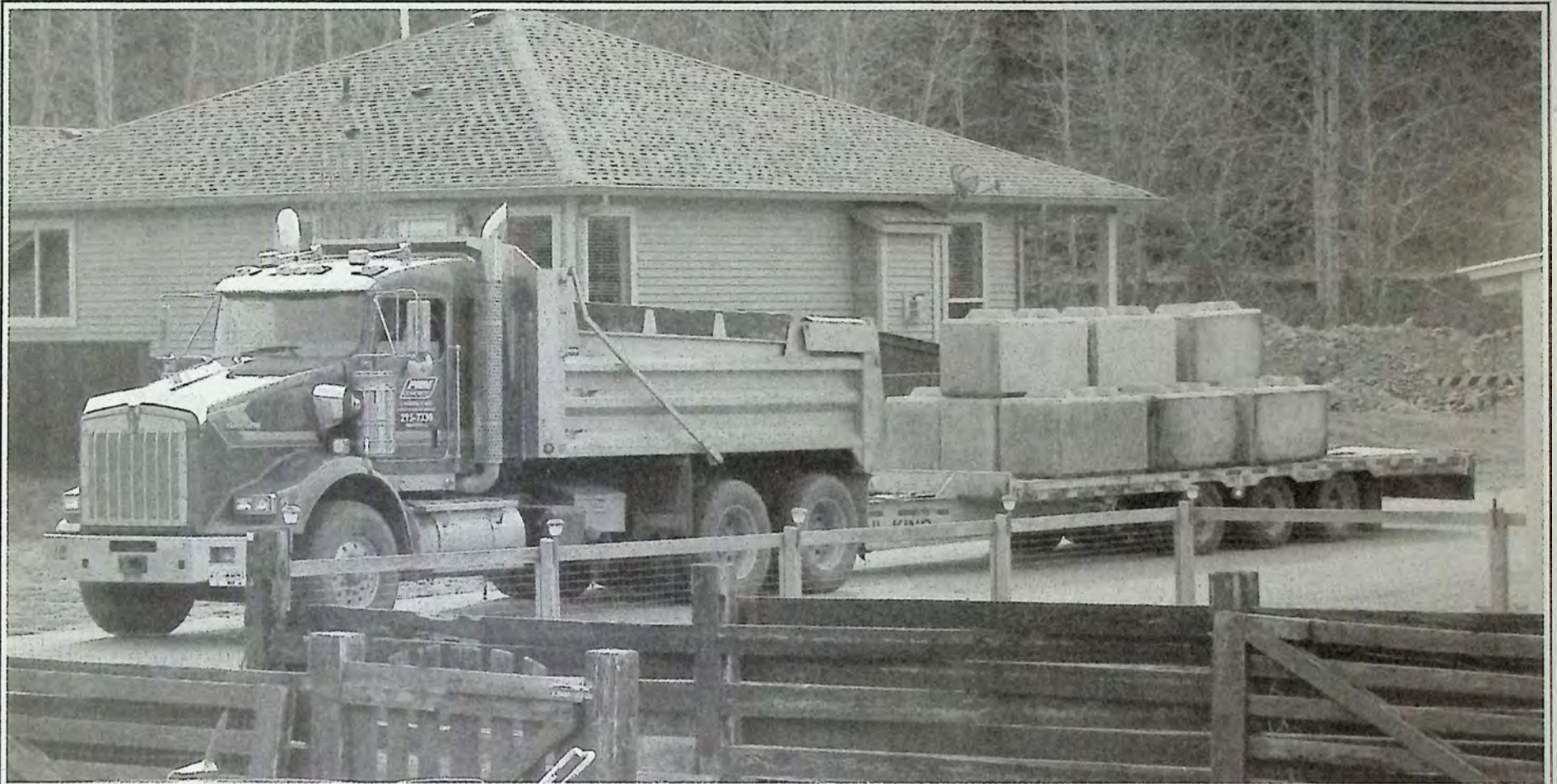
Cement blocks get delivered to the Similkameen River dike project as the Town of Princeton works to save other parts of the community. Photo: Brenda Engel
