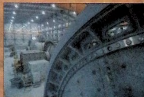
Once the secondary crusher is fully operational, the mine will be capable of processing ore consistently at its design capacity of 35,000 tpd.
