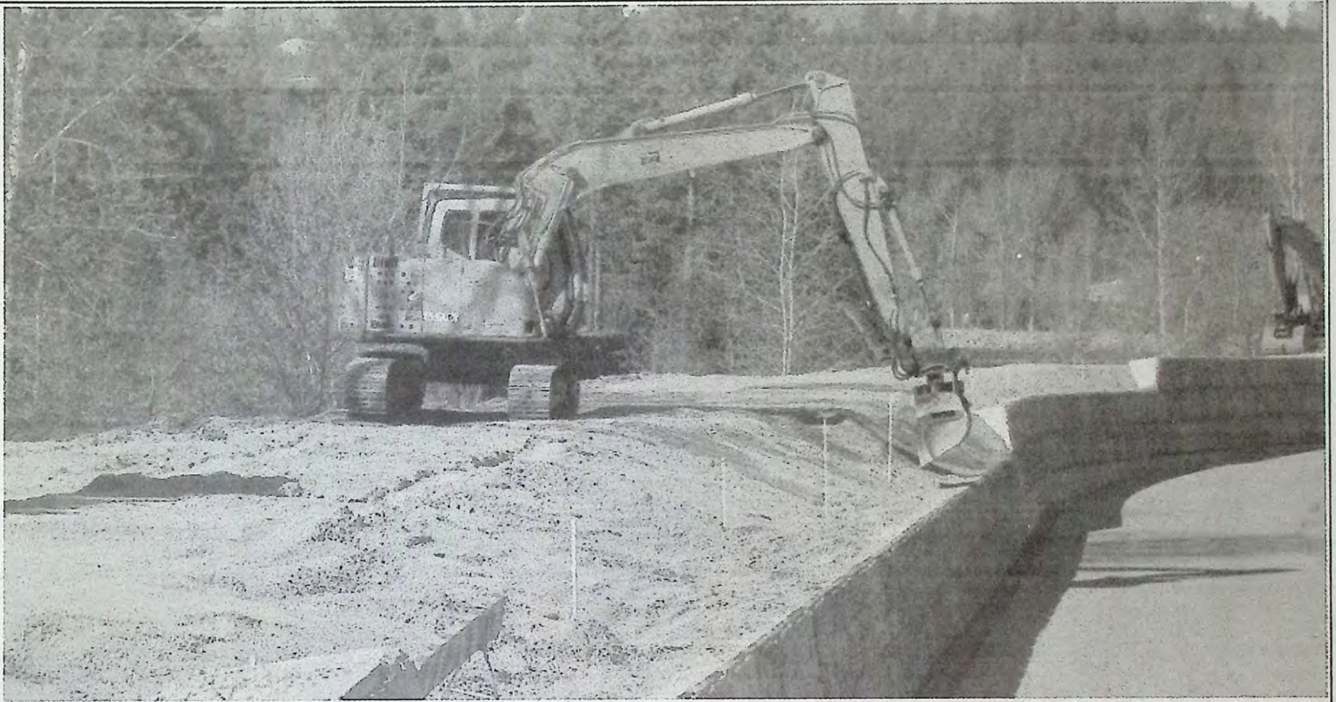
Dike improvements along the Similkameen River in Princeton are of interest to residents living downstream in communities such as Hedley and Keremeos. . Photo: Brenda Engel
