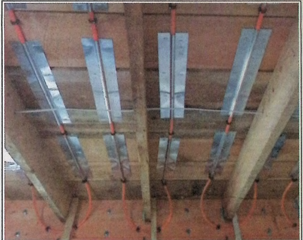
Under floor heating lines as viewed from below and looking up. One of many upgrades.
