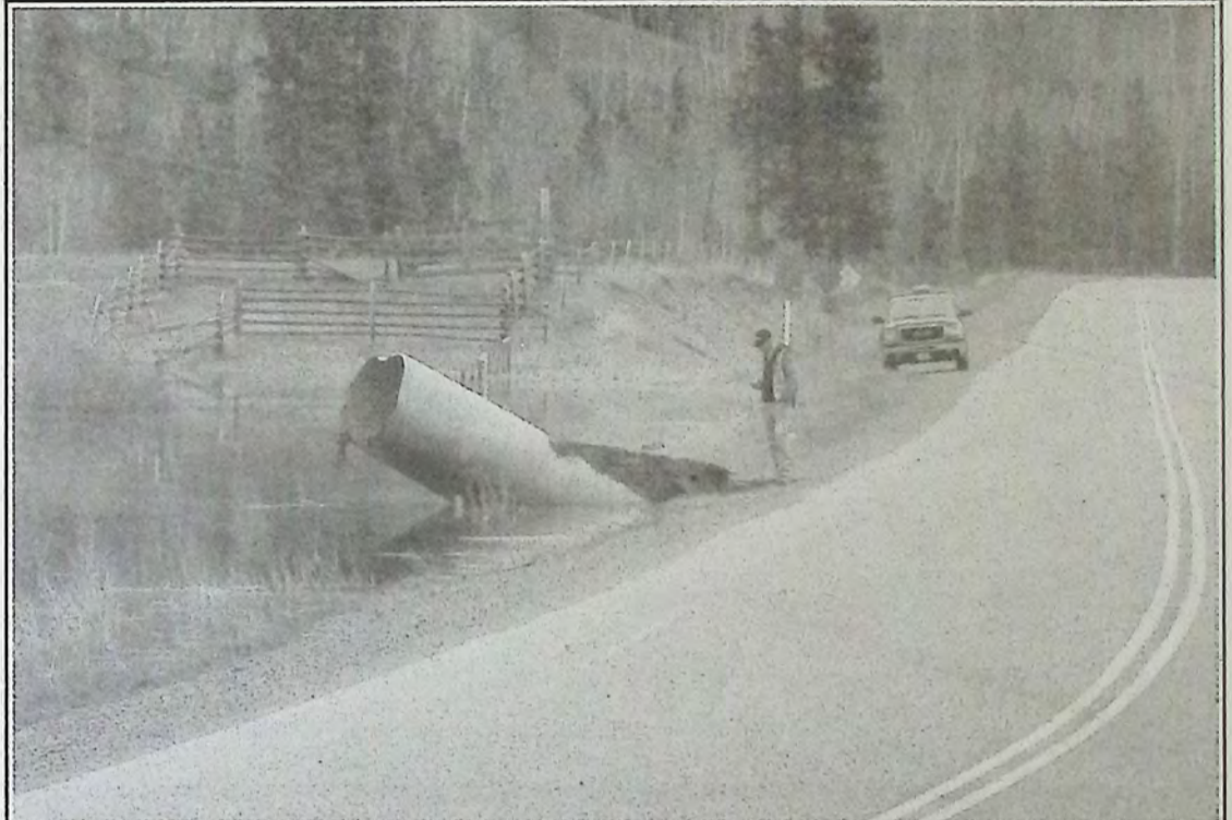
This drainage culvert was being examined by highways crew members early May 5th. It is located north of Princeton on Highway 5A near Aspen Grove. The worker in the photo told the News Leader that beaver activity created an 'air lock' in the culvert that forced it up out of the ditch in the same manner an air-filled bottle would. Photo: Brenda Engel
