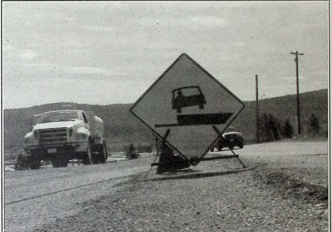
Expect minor delays on Old Hedley Road near the intersection with Highway 5A as a joint project repairs a short stretch of the road in the area. The project is expected to be complete by the middle of June. *
