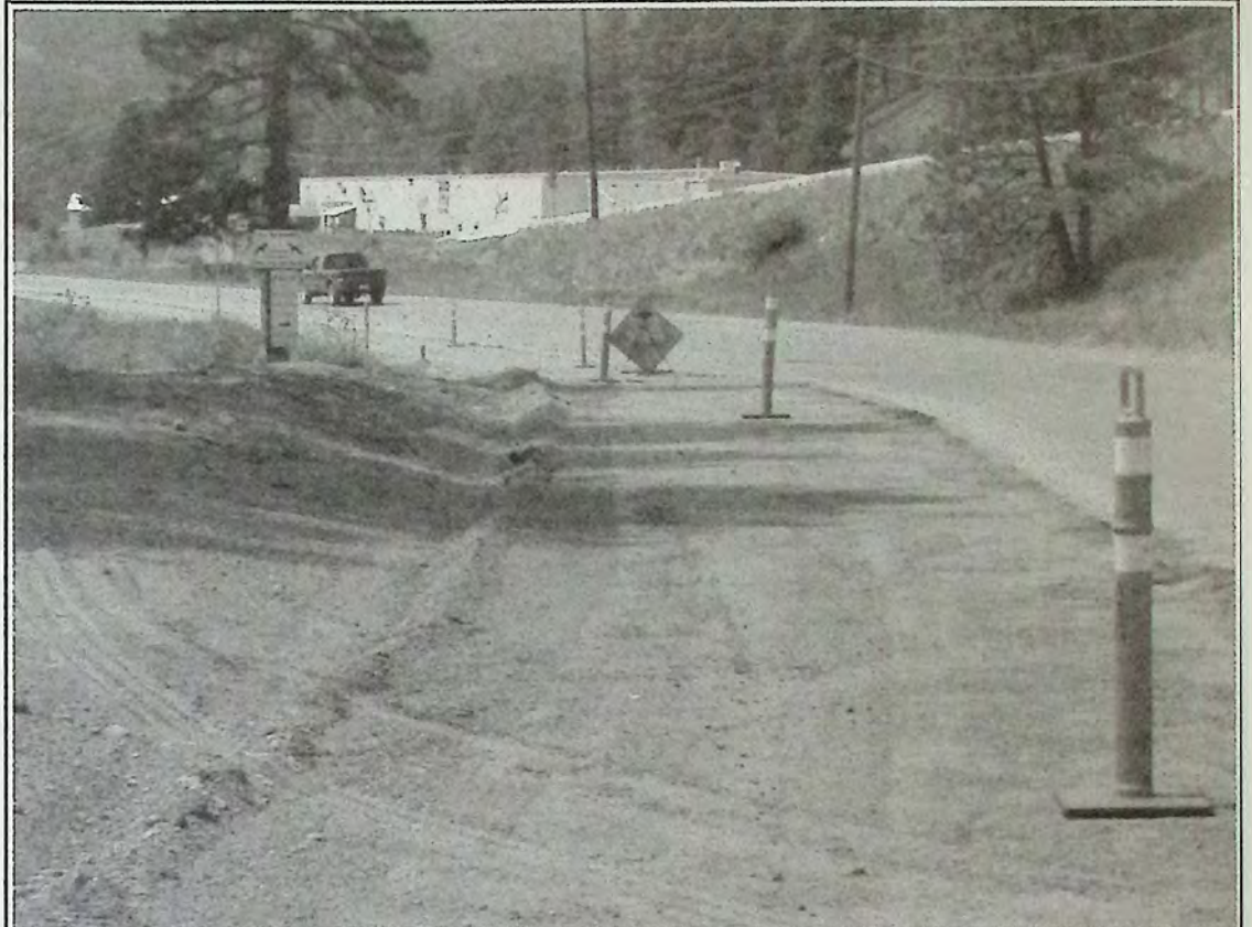
Repairs to Old Hedley Road started last week. The project, funded in part by the Town of Princeton, Weyerhaeuser and Princeton Co-Gen, will see improvements to the section of the road near those industrial sites. Photo: Brenda Engel
