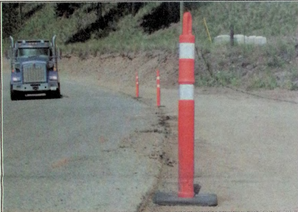
A $300,000 repair job to a section of Old Hedley Road is underway. The project, which will see a 4-inch surface along with other cosmetic changes (corner straightening, lane widening and intersection redesign), is jointly funded by the Town of Princeton, Princeton Co-Gen and Weyerhaeuser. Heavy truck traffic at those sites have made the repairs necessary. *
