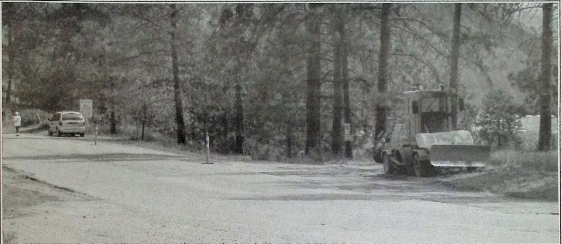
Crews were just getting set up along Old Hedley Road when we checked on the project early last week. Expect minor delays for a couple of weeks. Photo: Brenda Engel
