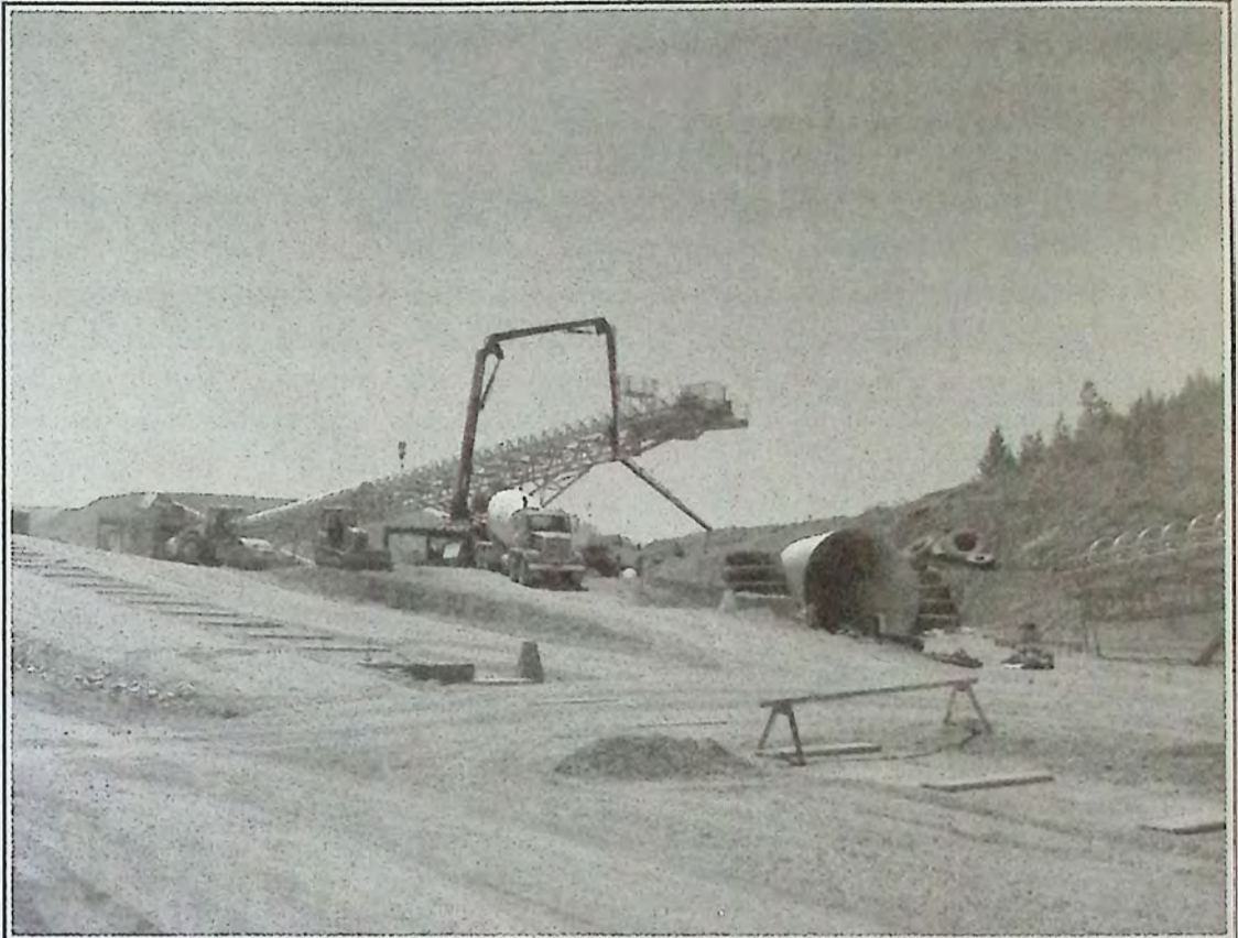
What looks like an unfinished maze of midair passages is actually part of a new conveyor belt system that will feed ore to the secondary crusher at Copper Mountain Mine and then will run the crushed ore along a ground level conveyor belt (which will sit on the cement footings in the foreground) to the SAG mill for further processing. *
