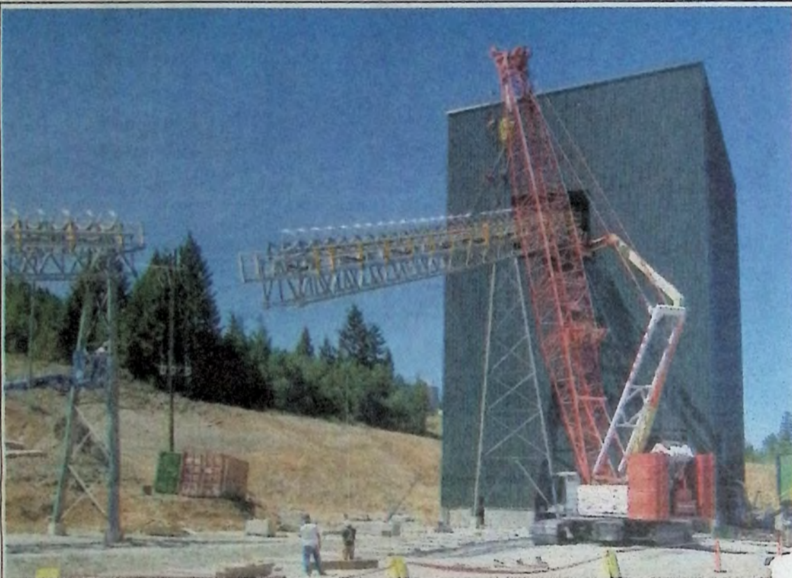
A 33-ton section of conveyor belt was lifted into place July 9th at Copper Mountain Mine. This was the largest single piece of the belt to be lifted and after a couple of rigging changes it was fit into place. The green building it feeds to houses the secondary crusher which will be operational later this year increasing productivity at the mine. *
