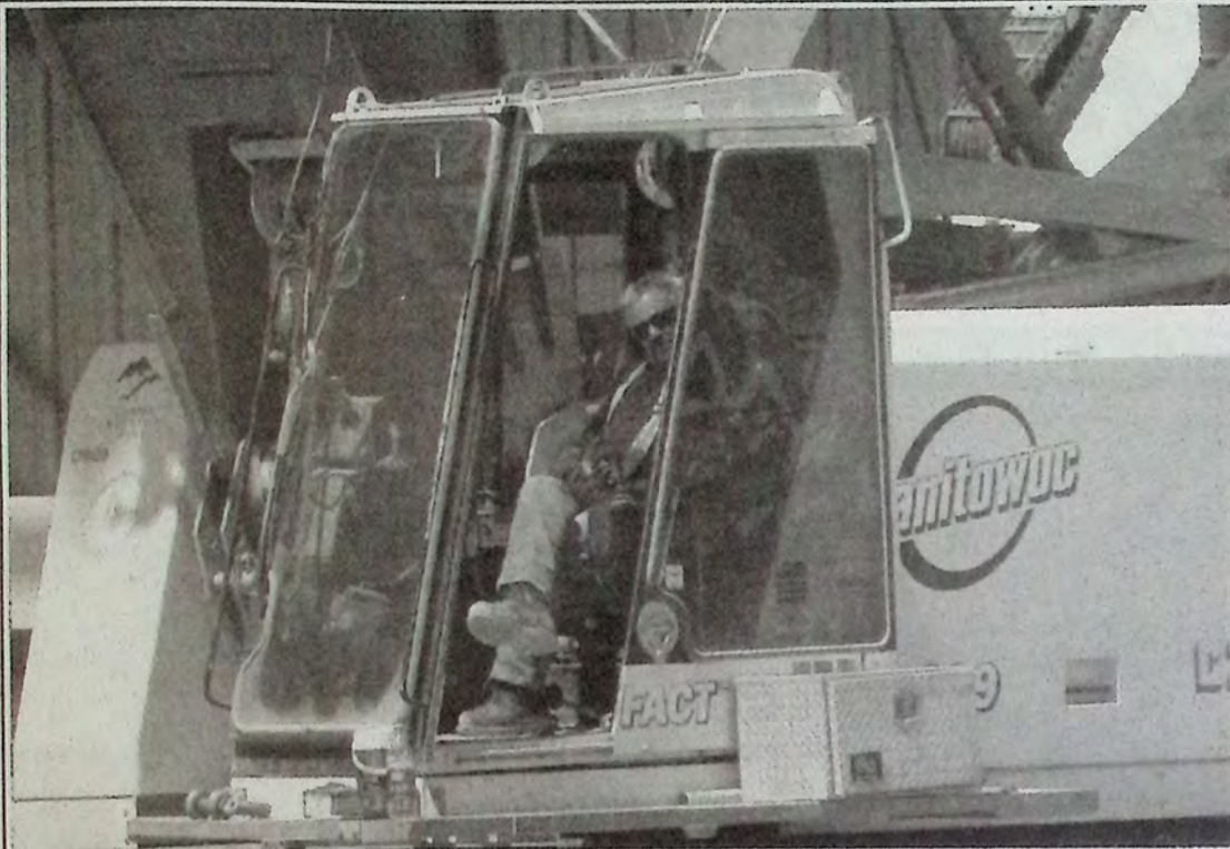
The man at the controls of the giant conveyor belt lift July 9th at Copper Mountain Mine was crane operator Grant Davies of Princeton. His steady hand and calm nerves completed the job without complication. *
