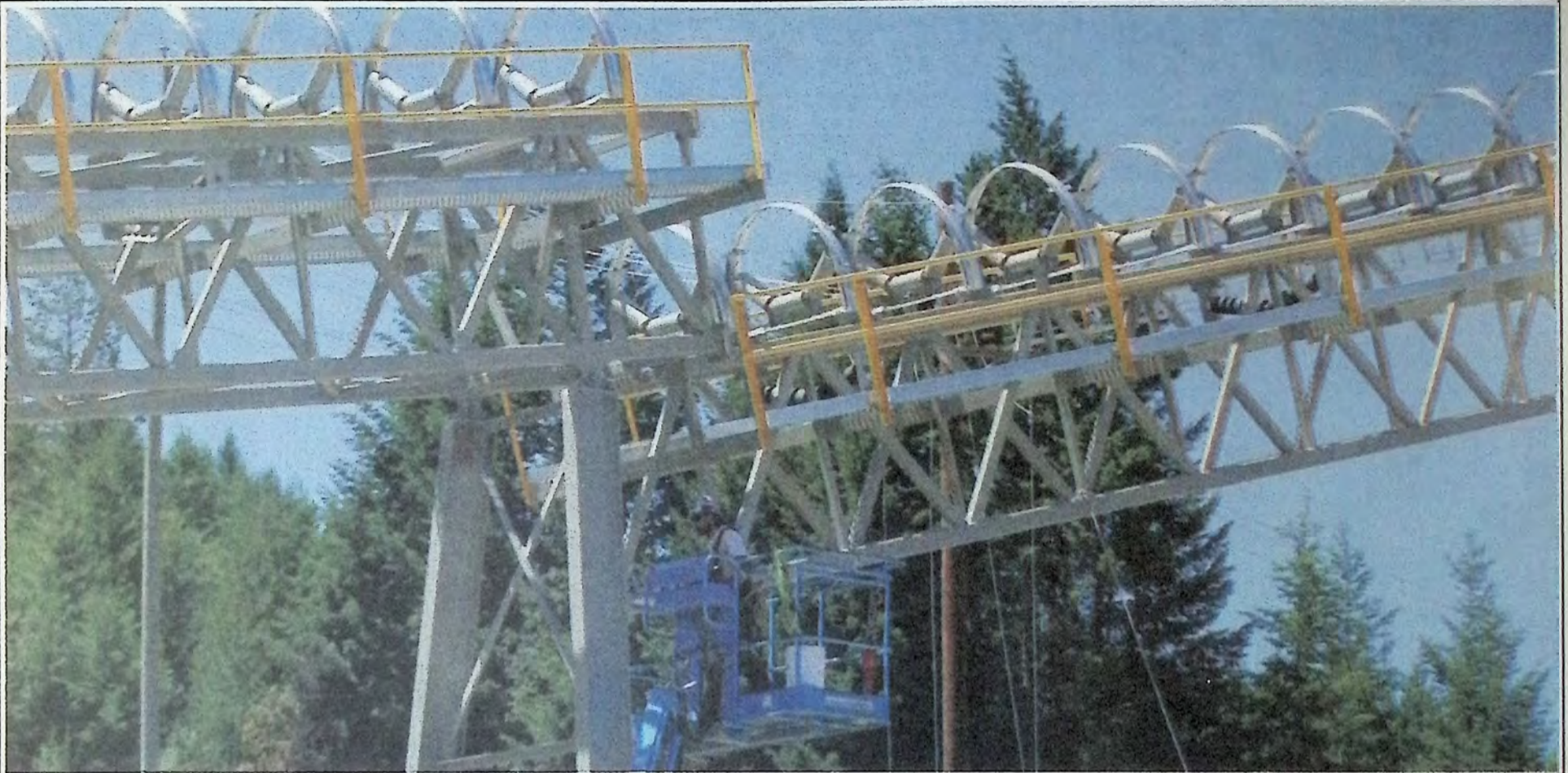
An up close look at one end of the conveyor belt lift project July 9th at Copper Mountain Mine. *
