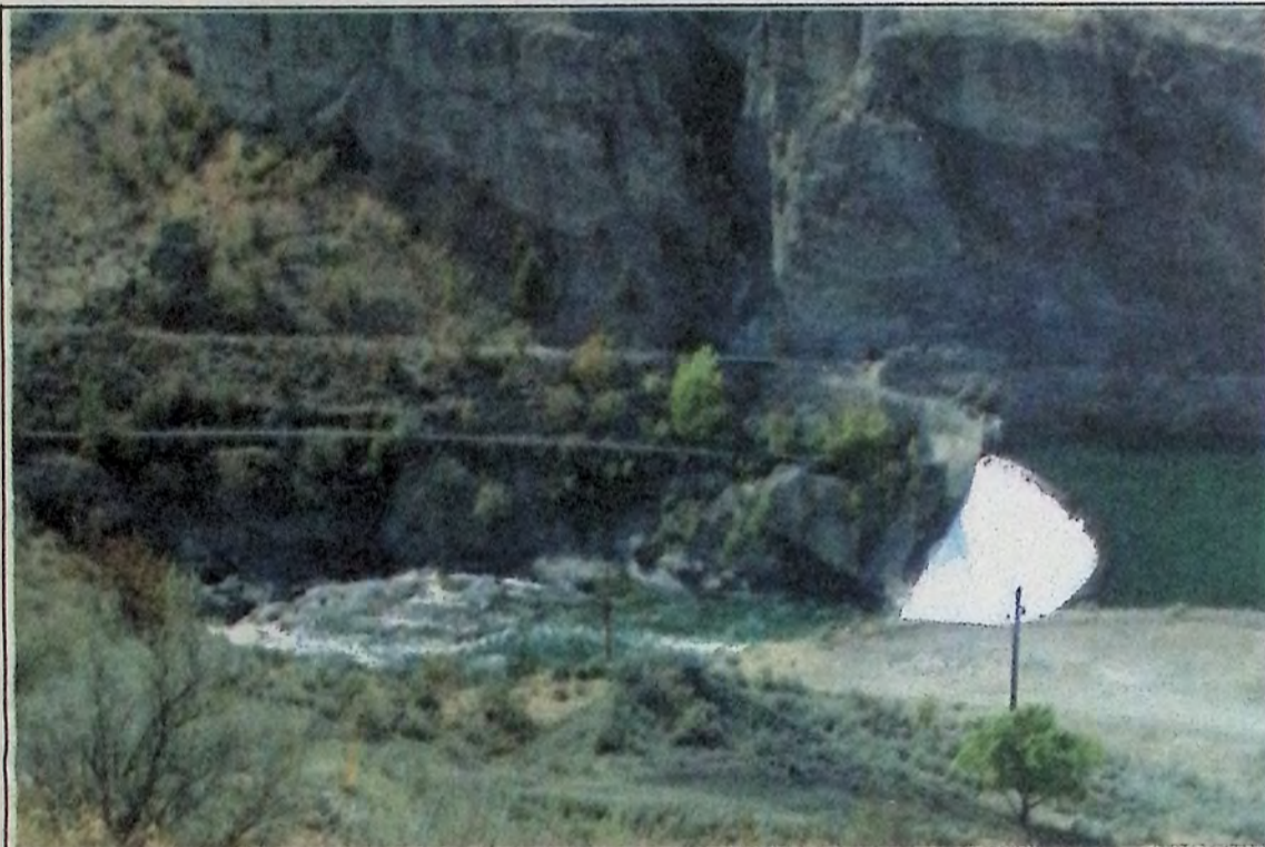
The Enloe Dam, which opened in 1920, is located just above the US Similkameen Falls (the top is visible in the left of this photo) and has not been operational since 1958. This was how it looked last week from Enloe Dam Road. *
