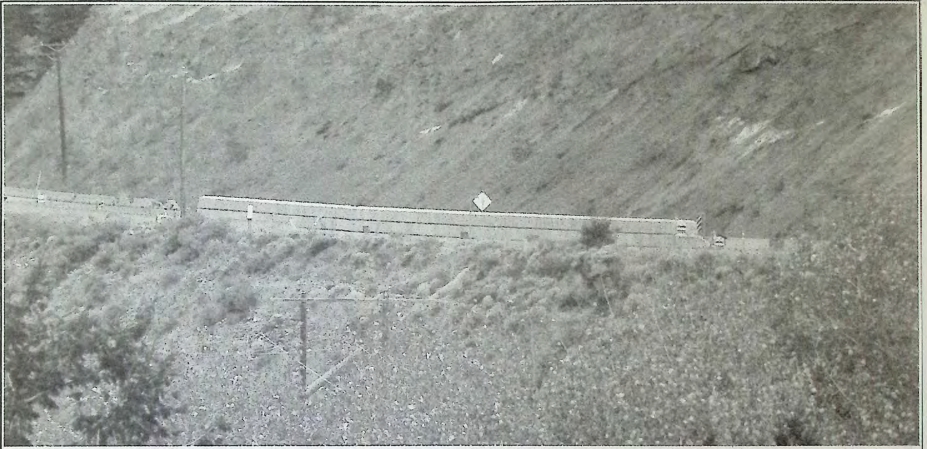
This is how the repair work on Highway 3 9-kilometres west of Keremeos looked last week. Photo: Brenda Engel
