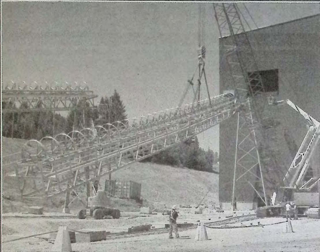
A feeder line installed during the summer allowed Copper Mountain Mine to add a secondary crusher to their production line. The conveyor belt lift went smoothly following a lengthy delay on site. *
