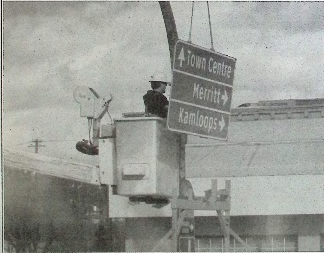
Old, outdated and weathered highway signs were removed and replaced by newer ones along the Highway 3 and Highway 5 corridors within the Town of Princeton. They were long overdue. Photo: Brenda Engel
