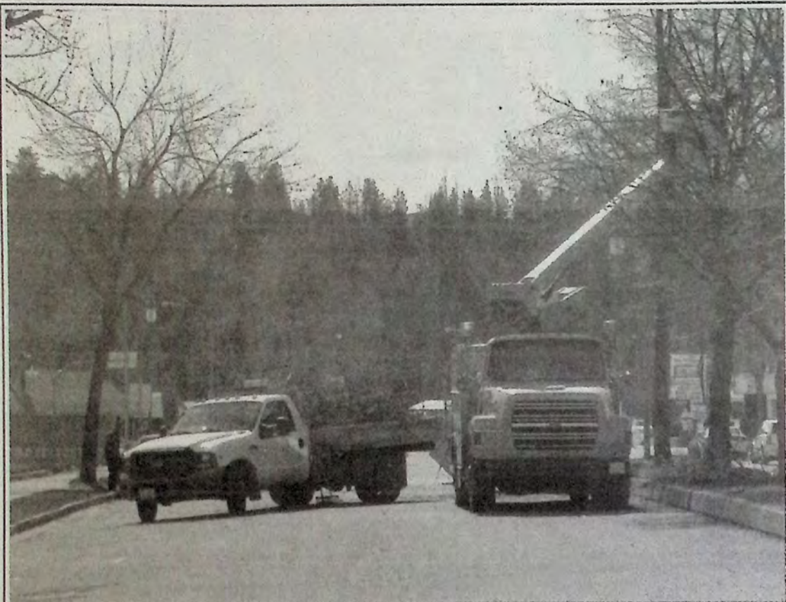
Spring has arrived and the Town of Princeton Public Works Department has been busy on various clean up jobs around the community. We found them pruning on Vermilion Avenue late last week. *
