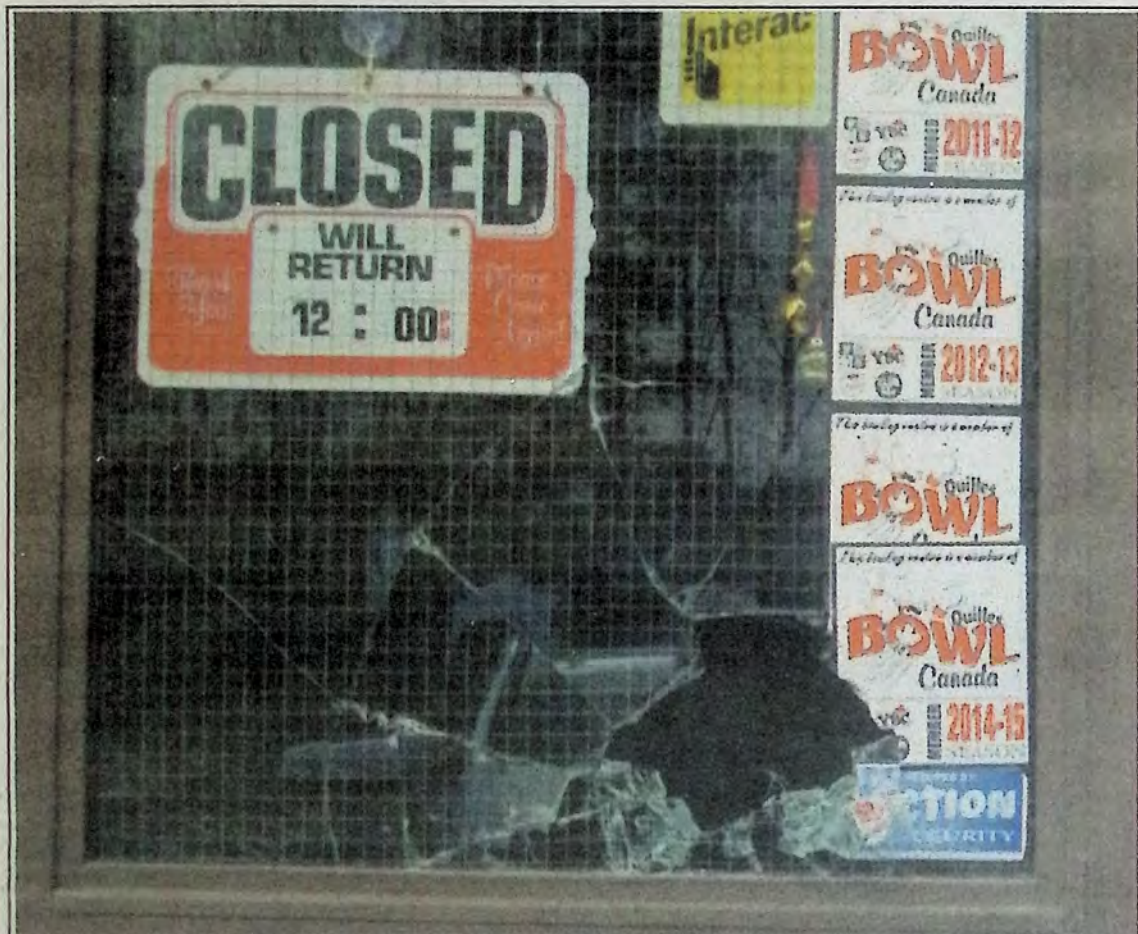
Safety glass in the front door window at Copperhill Lanes would have taken time to have broken in order to enter the premises. If you heard anything March 31st you are asked to contact RCMP at 250-295-6911. - photo submitted
