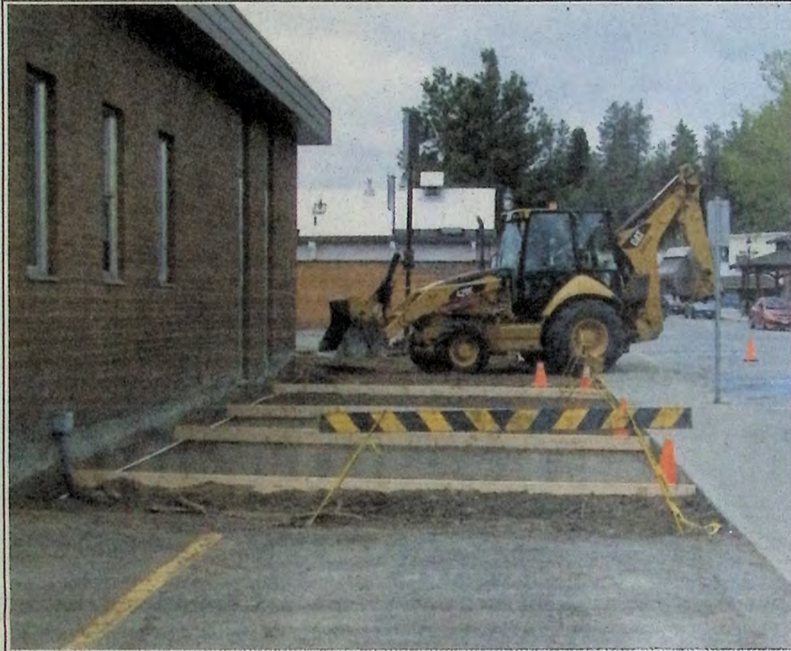
The Town of Princeton InfoCentre is taking shape daily. Last week was spent preparing the lawn area for paving stones and grass before the installation of picnic tables. Exterior painting was also completed as part of the project. *
