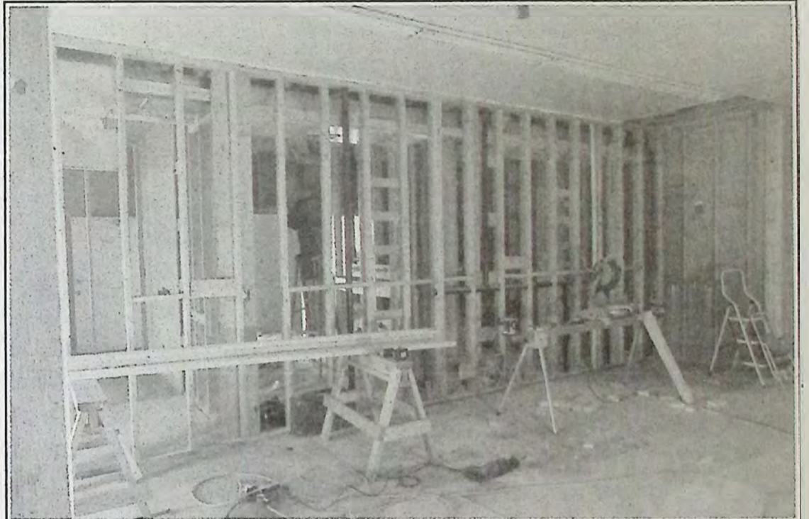
This was once the kitchen area at the former 'pub on the hill' and is slowly being transformed into change rooms and office space for the soon-to-open LivinIt Fitness centre. Through the wall is washrooms that are being redesigned. *
