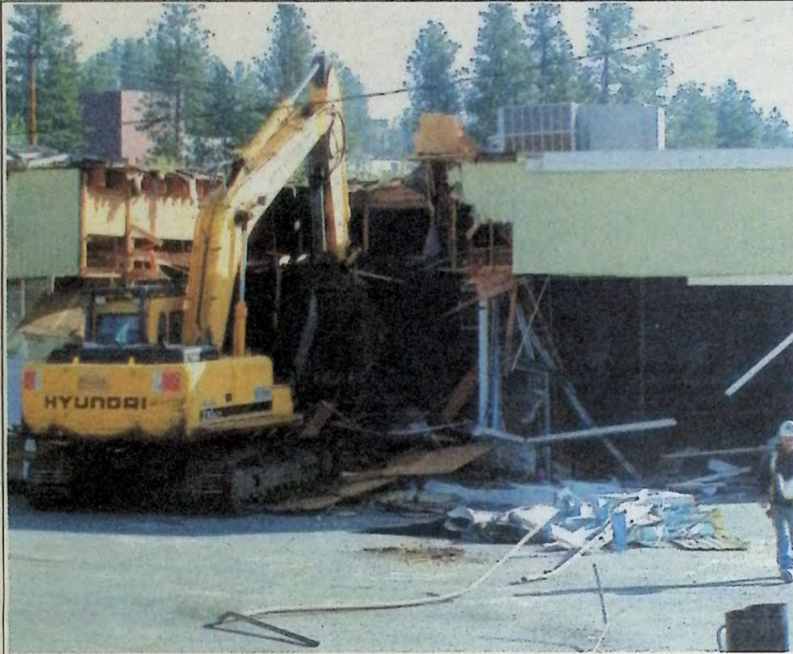
Demolition of the former Overwaita Foods building on Bridge Street started at 8:00 AM on Friday, May 8th. The building has sat empty since the new Cooper's Foods grocery store opened across the street a few years ago. *
