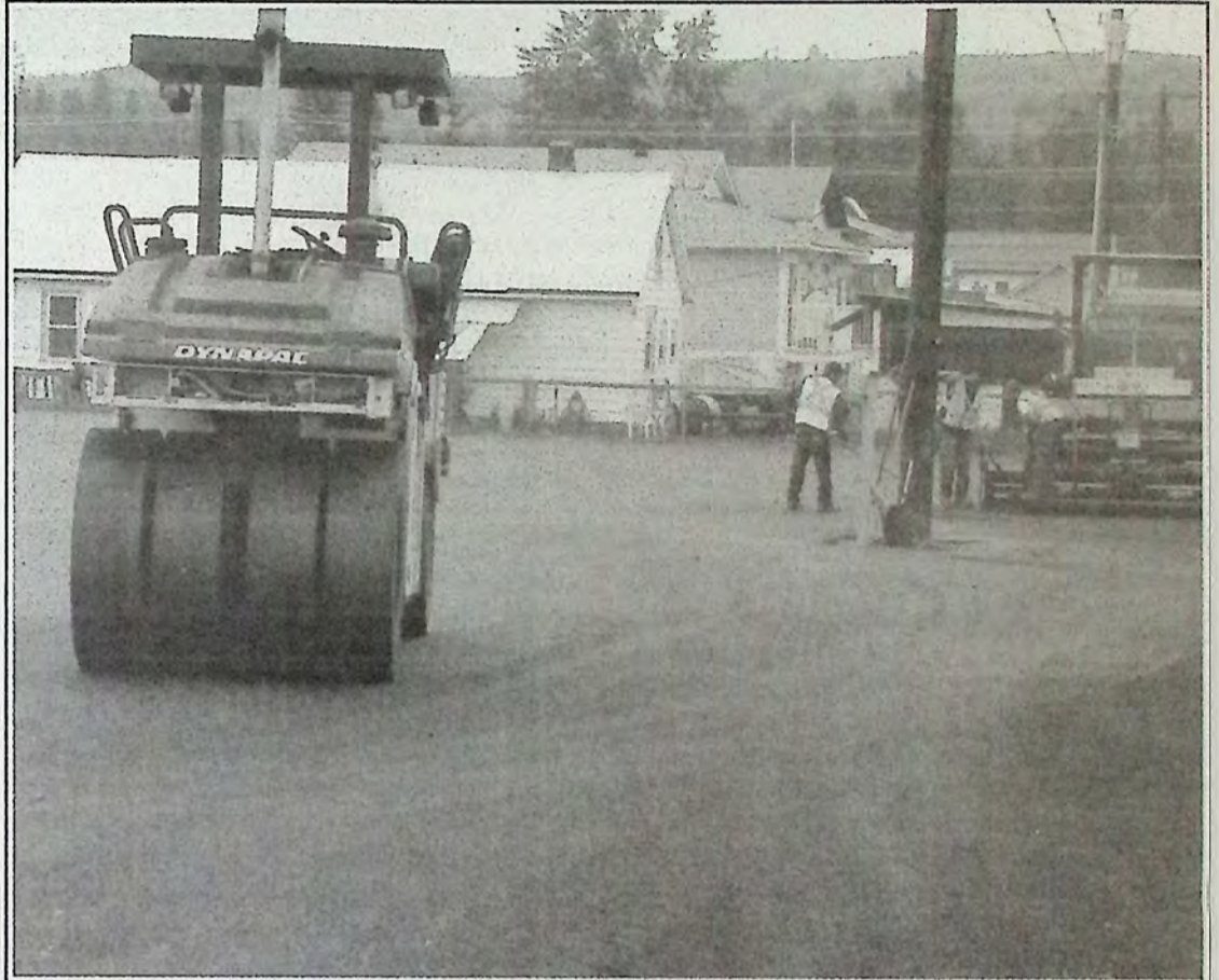
Parking lot and alley paving took place last week as the Town of Princeton nears completion on the new tourist information centre which will be located in the downtown core in the former town hall building.*
