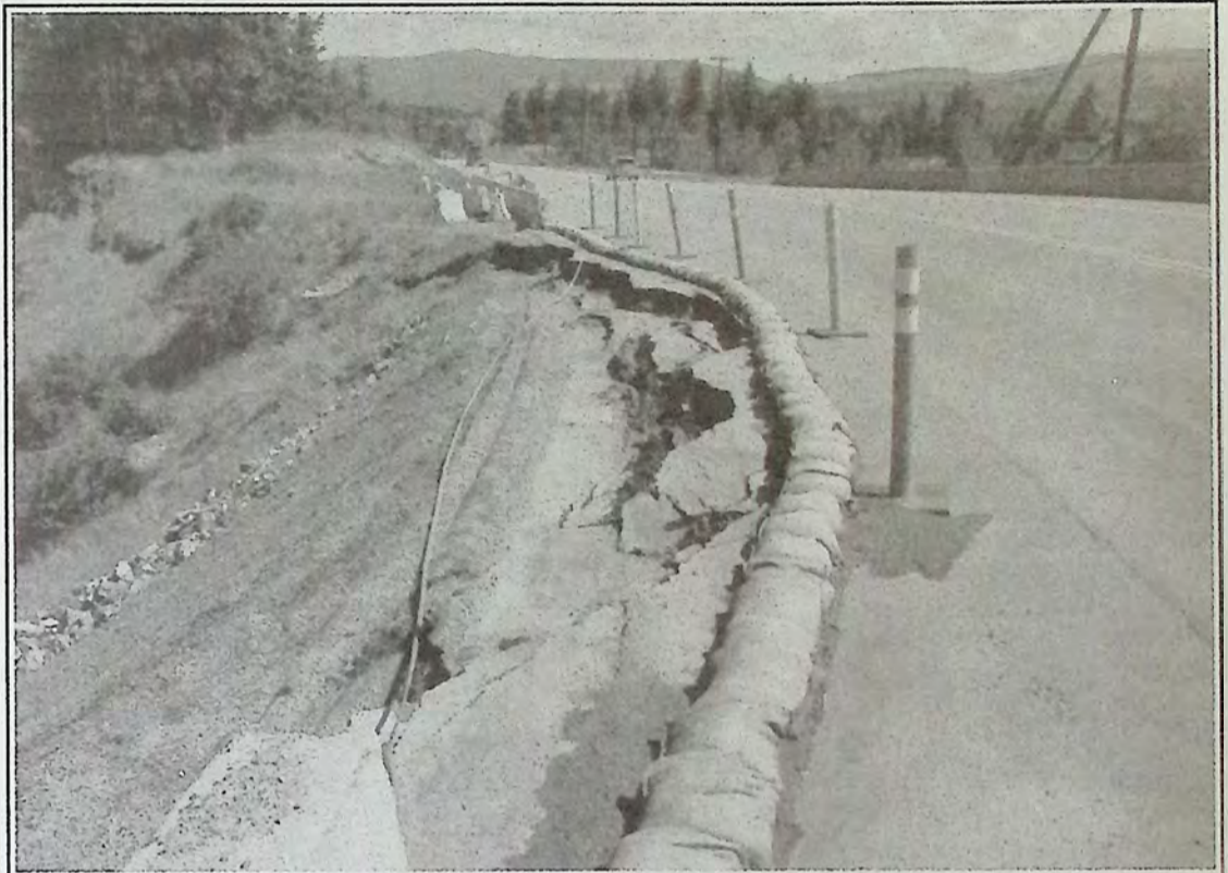
It must be spring as part of Highway 3 just west of Princeton is starting to disappear...again. *
