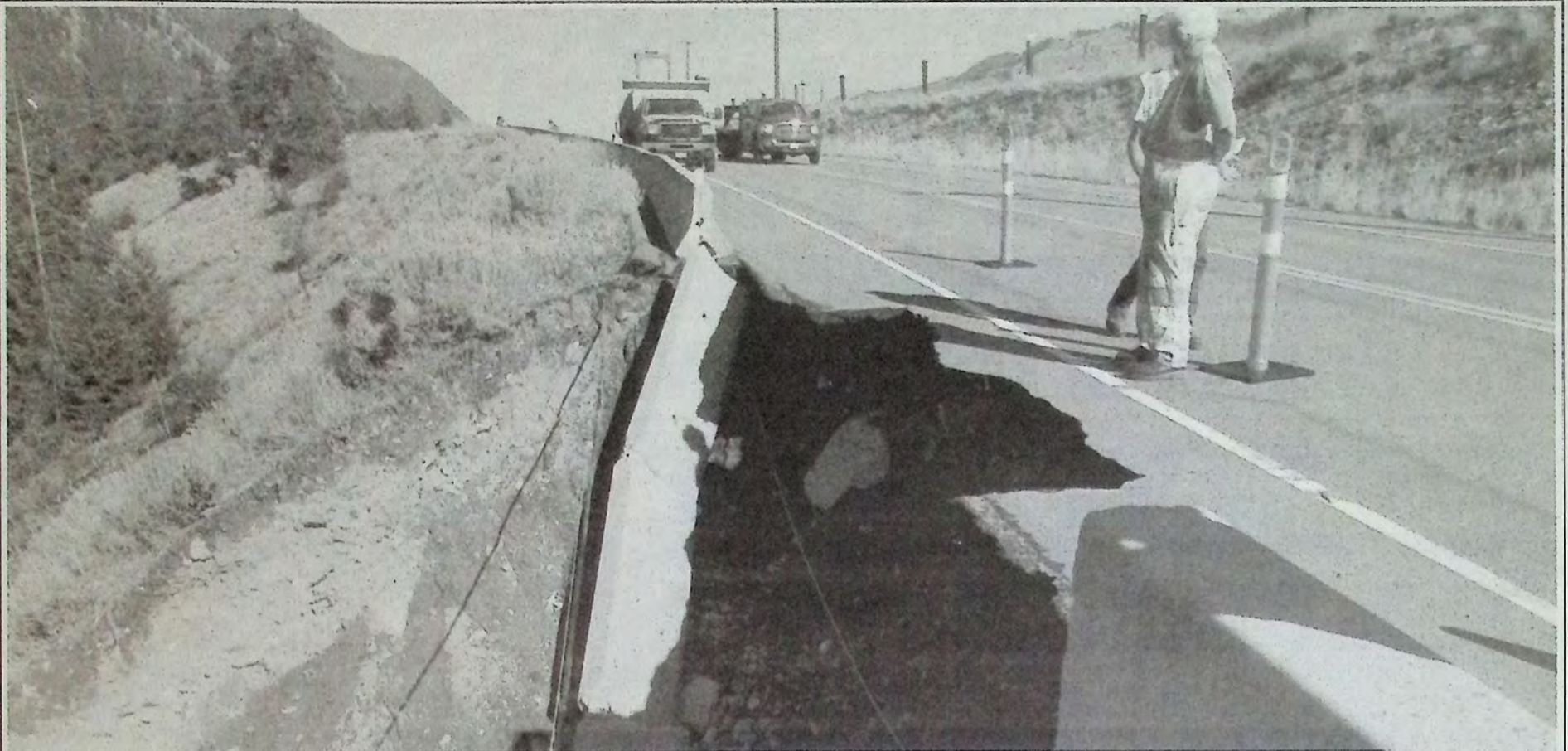
Heavy rain that passed through Hedley and Keremeos damaged a piece of Highway 3 2-kilometres East of Hedley July 20th. Crews fixed it by midday. *
