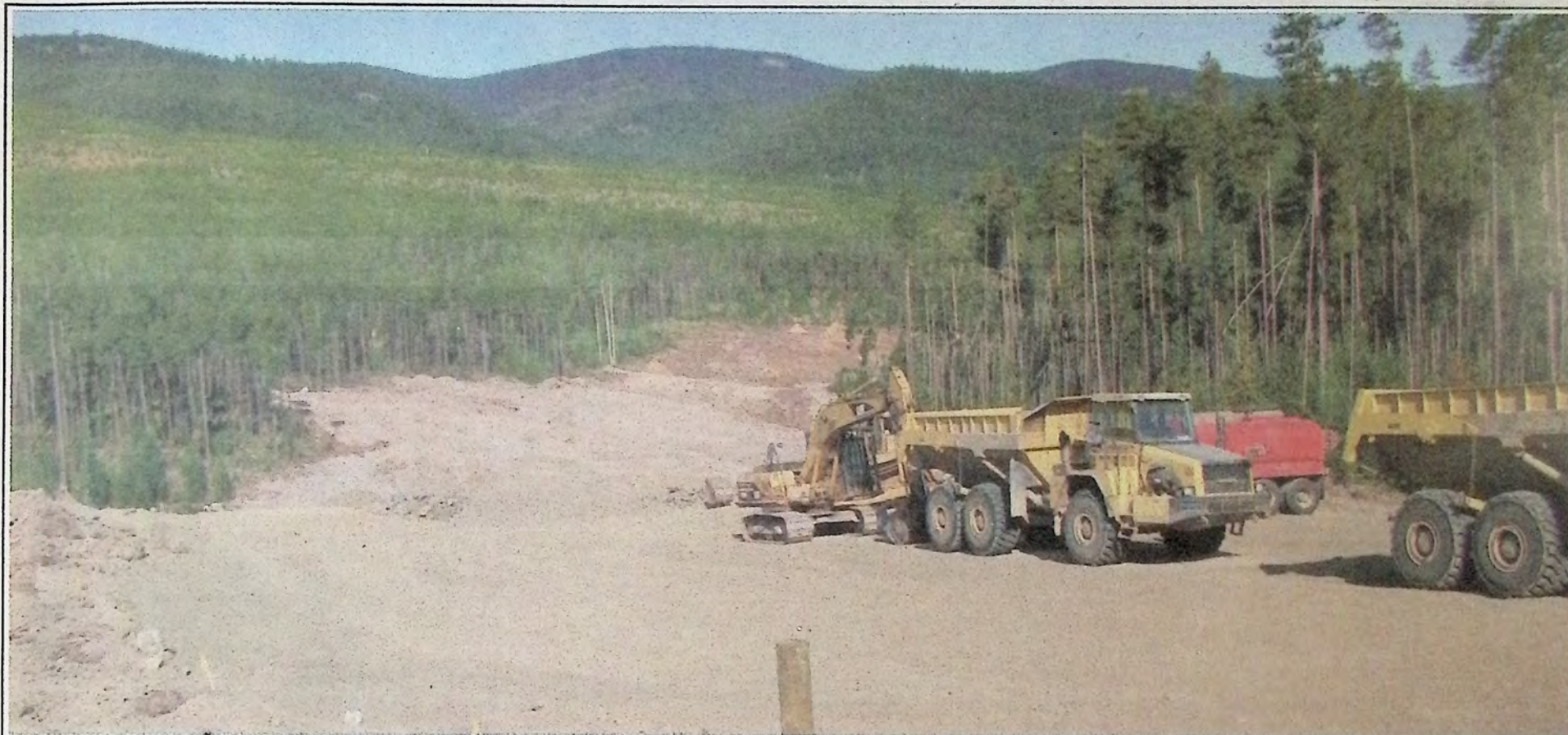
Near Sunday Summit you can clearly identify the proposed path that Highway 3 will take to eliminate another sharp corner on the route. Clearing for the roadway continues on this project. *
