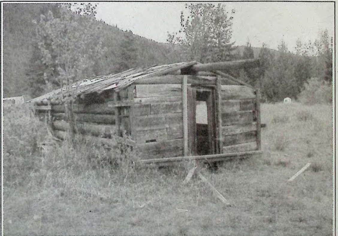
The only building still standing in the Granite Creek townsite is this one. *
