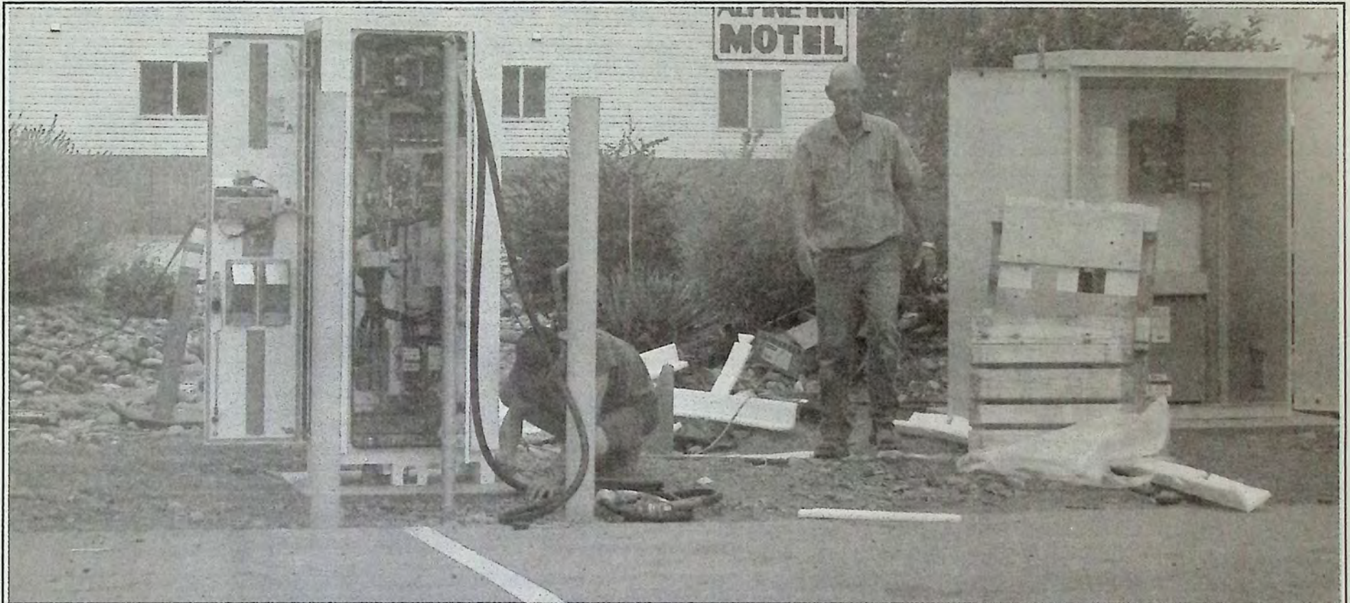
Dane (crouched) and Ken (standing) from PowerTrend Electric Ltd. were busy installing the new electric charging station in Keremeos August 24th. The Keremeos charging station is a collaborative effort between the Province of BC and BC Hydro. A robust DC charging system can recharge a car in 30 minutes. 100% plug-in electric vehicles need an electrical grid to recharge. Plug-in hybrid electric vehicles have a rechargeable battery plus an internal combustion engine. Powertech Labs - a subsidiary of BC Hydro - tracks usage across the province. In August 2013 there were 1,684 monthly charging sessions in BC. By August 2014 there were 3,745 monthly sessions, an increase of 120%. Visit www.fleetcarma.com/evcloud to see overall usage trends or your own vehicle usage. Photo: Arlene Arlow
