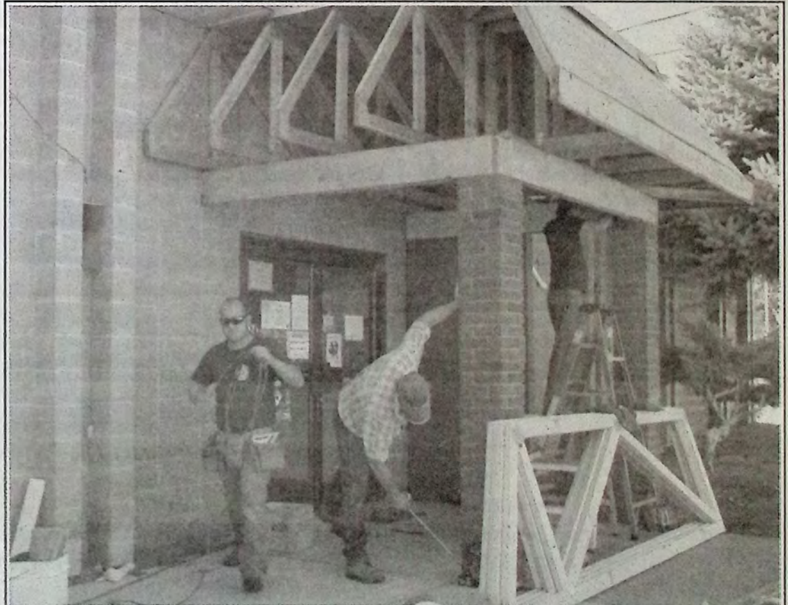
D'Arcy, Scott and Mark were busy ripping and tearing at the front of the Keremeos Seniors Hall October 13th. The trio is building a much-needed overhang at the front of the hall so that scooters can be kept out of the elements while their owners are inside. Photo: Arlene Arlow
