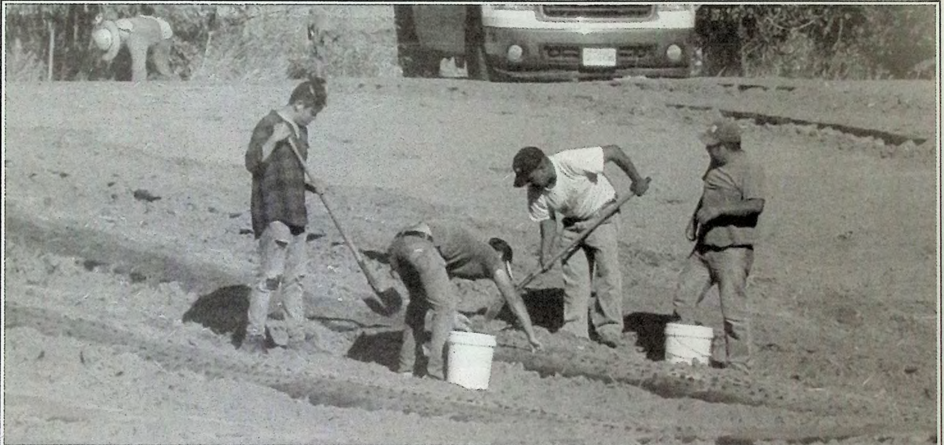
"You work hard for your money." This crew was installing rows of black plastic mulch along Highway 3 near Keremeos recently. The black plastic will be buried with dirt for the winter so that it doesn't weather too much. Come next Spring, ground crops will emerge from slits cut into the plastic. Plastic irrigation tubing inside the rows will ensure water isn't wasted due to evaporation. Photo: Arlene Arlow
