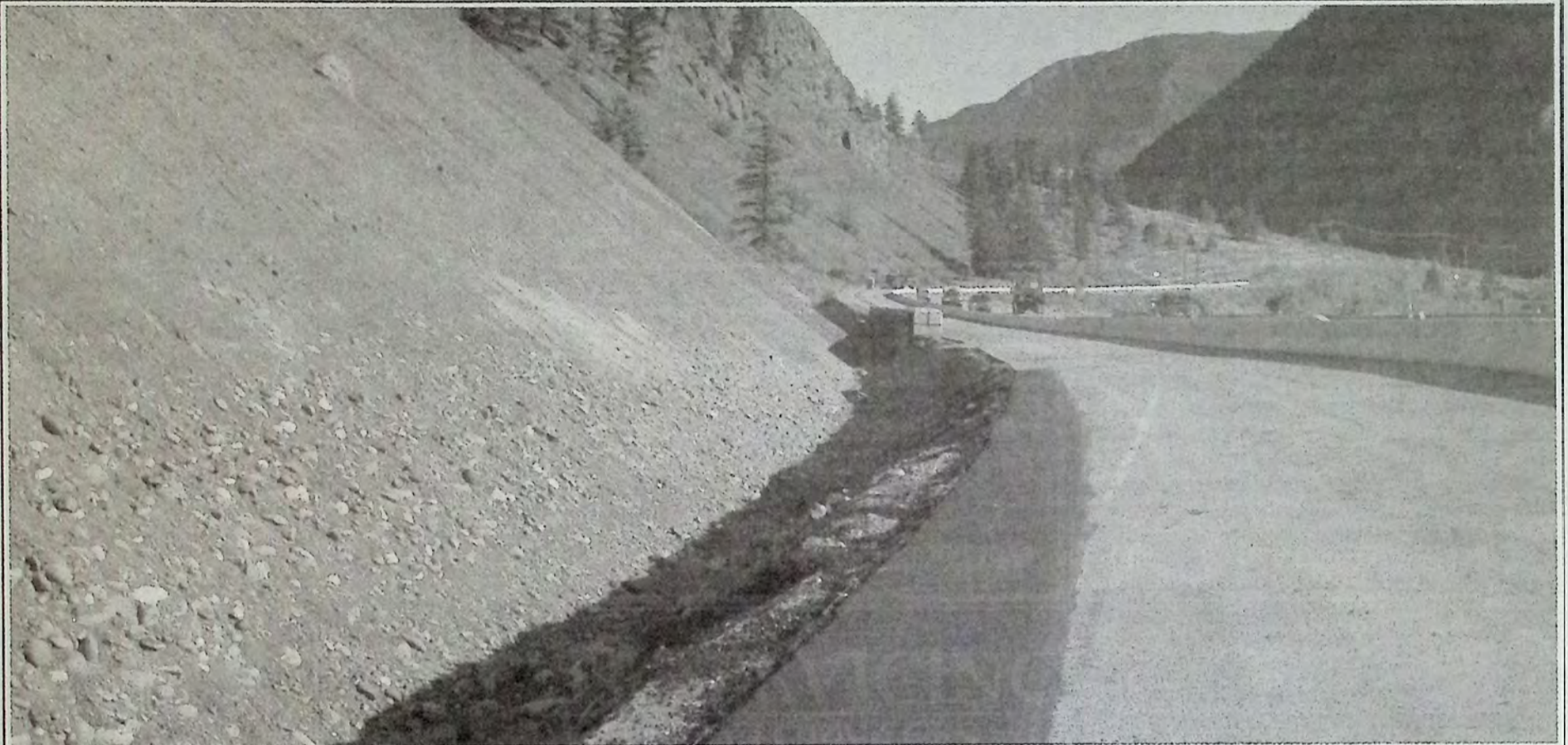
Based on the fact that there is no heavy machinery along Highway 3 west of Keremeos, it seems the ditch is done. The shoulder of the highway has been repaired and the only signs of a construction site are a port-a-pottie, an empty dump trailer and cement barricades. Photo: Arlene Arlow
